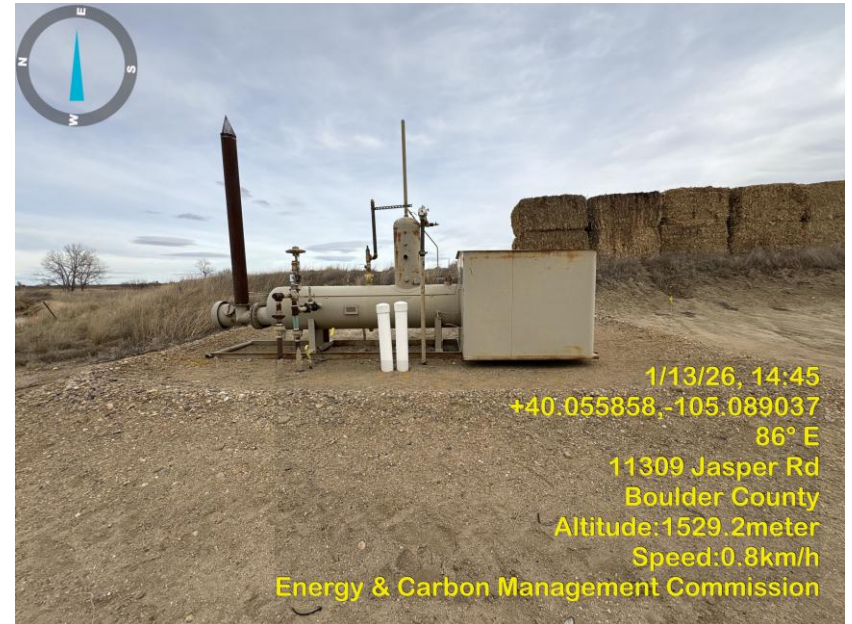
Photo 8 Horizontal Heated Separator.
