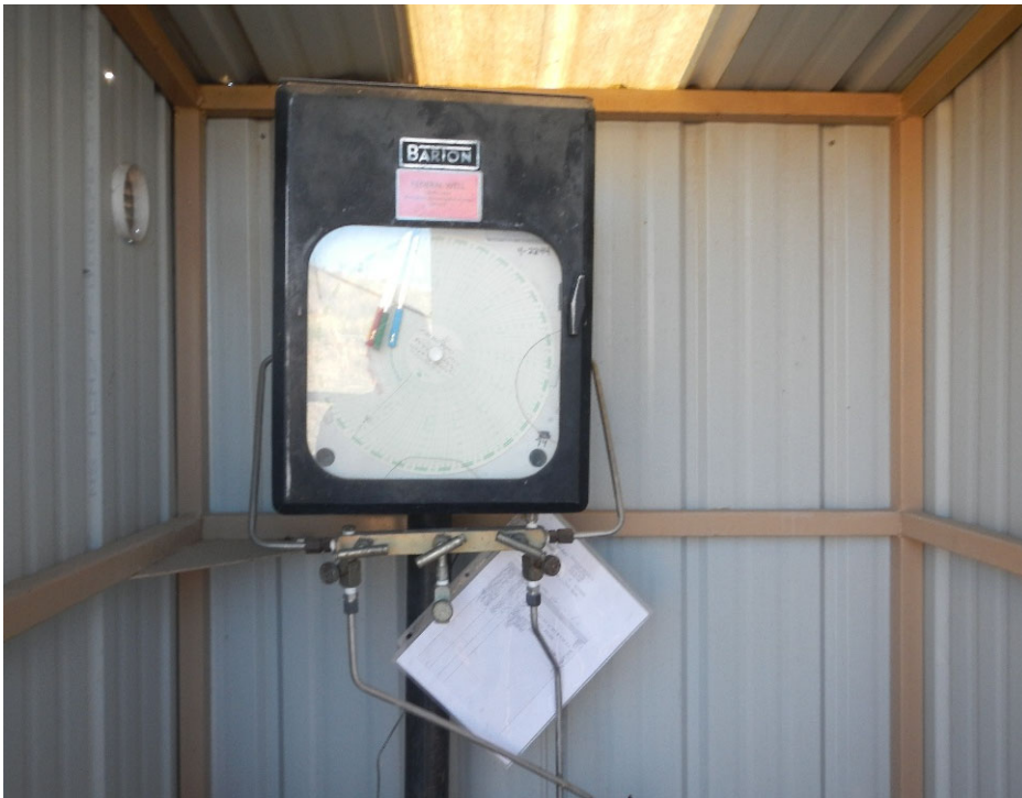
3. Gas Meter inside Meter Shed.
