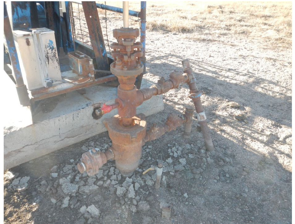
2. View of wellhead.
