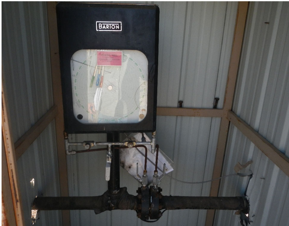
3. Gas Meter inside Meter Shed.
