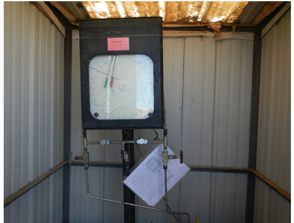
4. Gas Meter inside Meter Shed.
