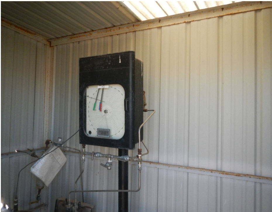
5. Gas Meter inside Meter Shed.
