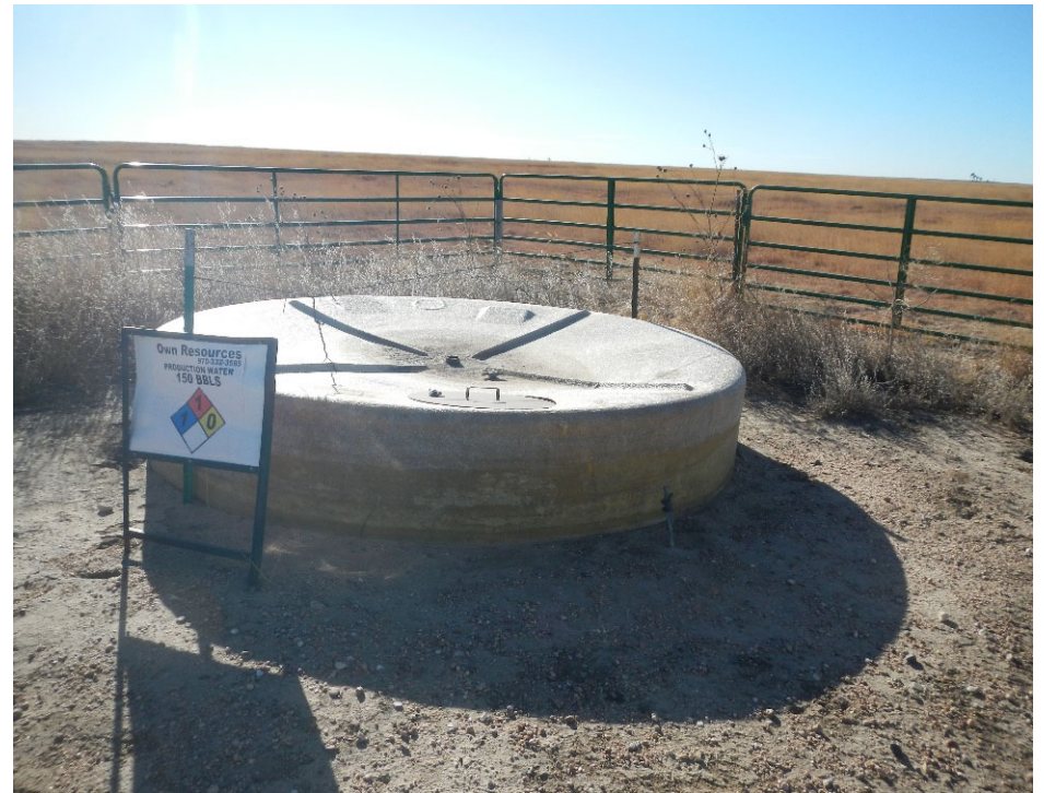
6. View of produced water tank at remote gathering location.
