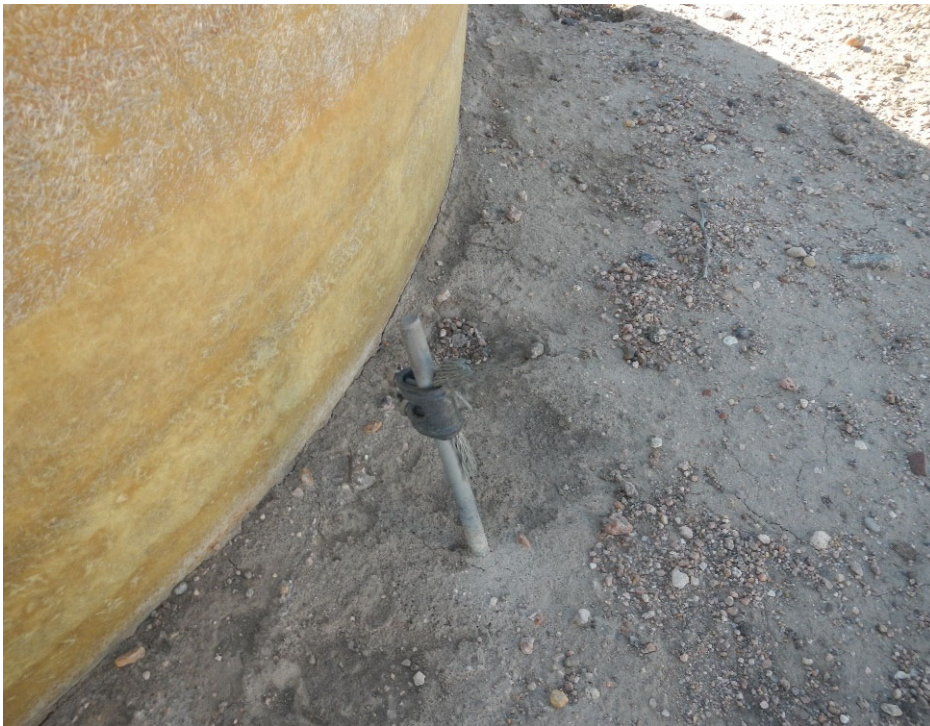
7. View of broken ground strap on production tank.
