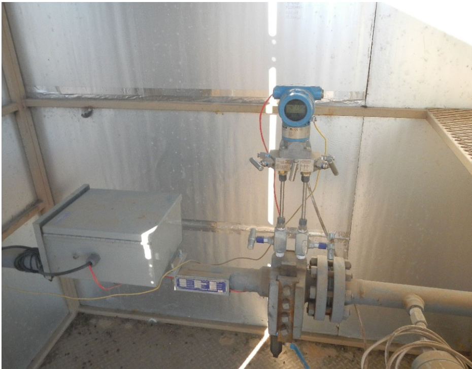
5. Gas Meter inside Meter Shed.
