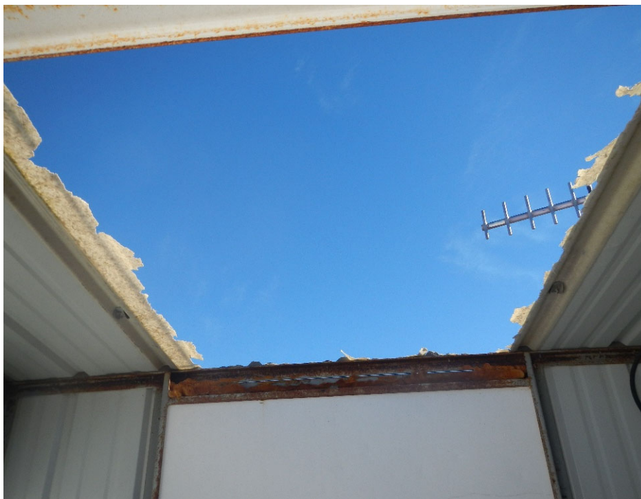
7. Roof damage on Gas Meter Shed.
