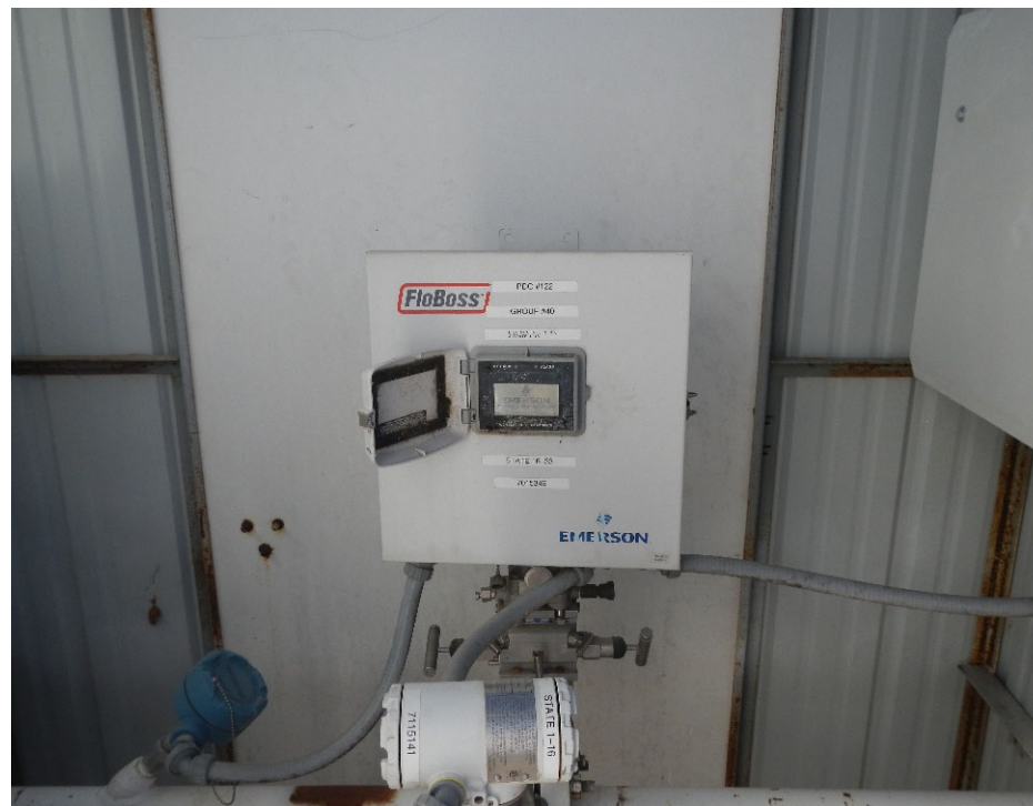
8. Gas meter inside shared meter shed.
