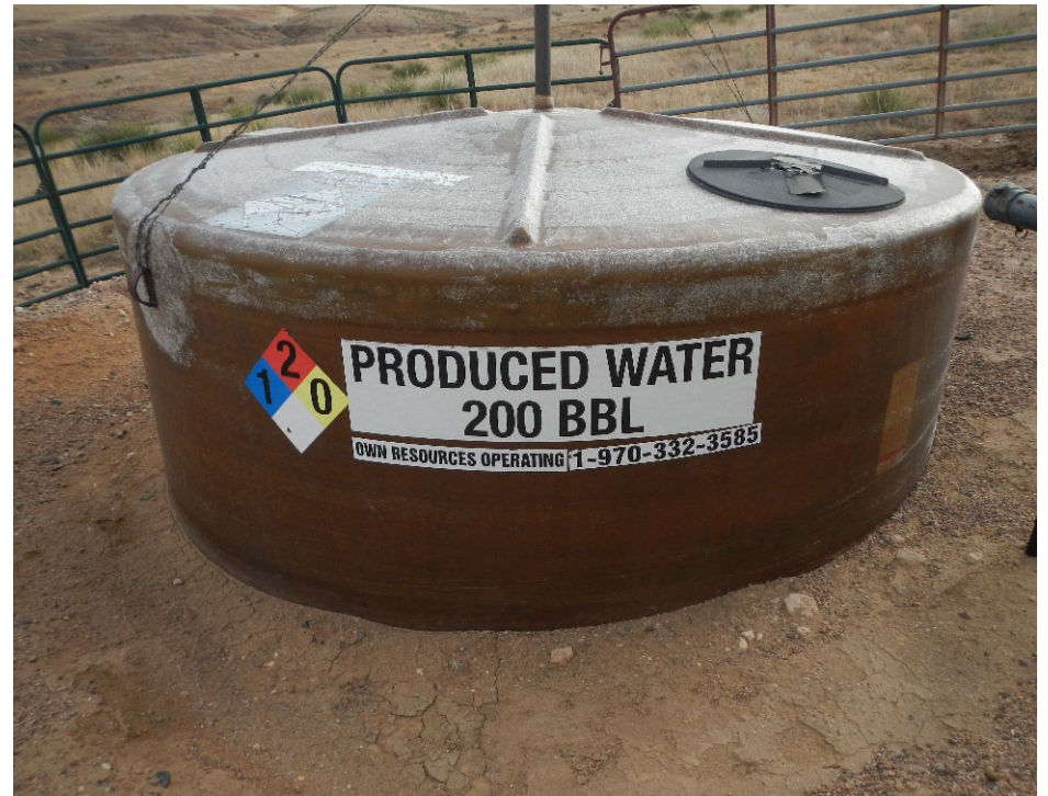
4. View of Production tank at well location.
