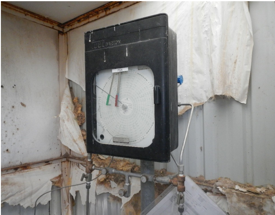
3. Gas Meter inside Meter Shed.
