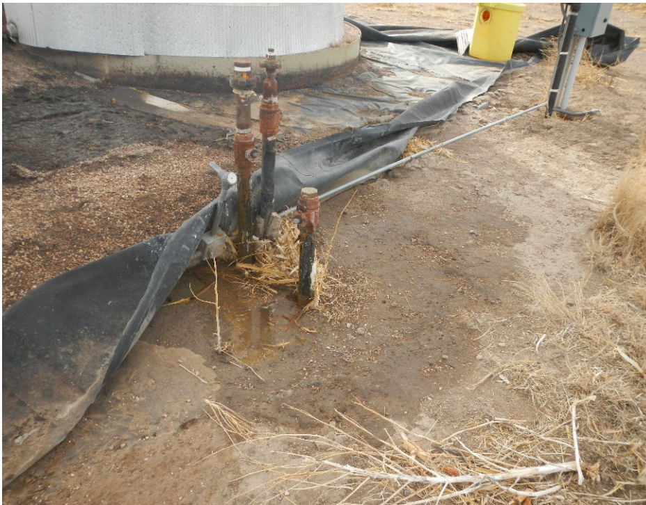
9. Additional view of flowline risers and fluid release around piping and under liner.
