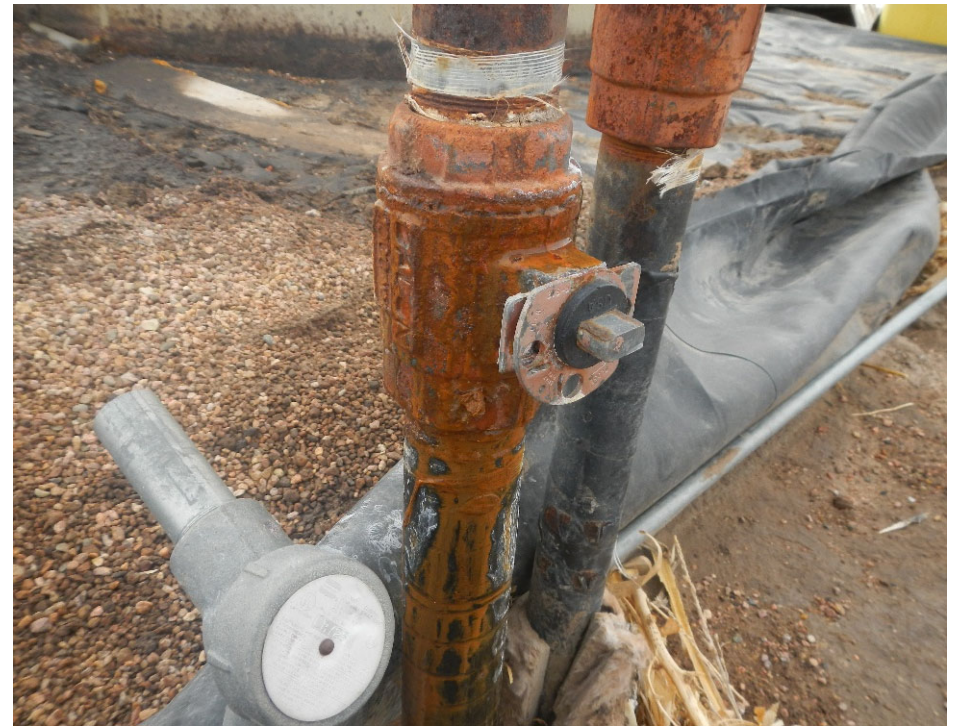
10. One of two flowline risers leaking from valve body and flowline to valve connection.
