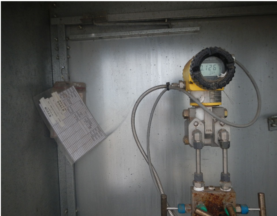
3. Gas Meter inside Flowline mounted Meter Box.
