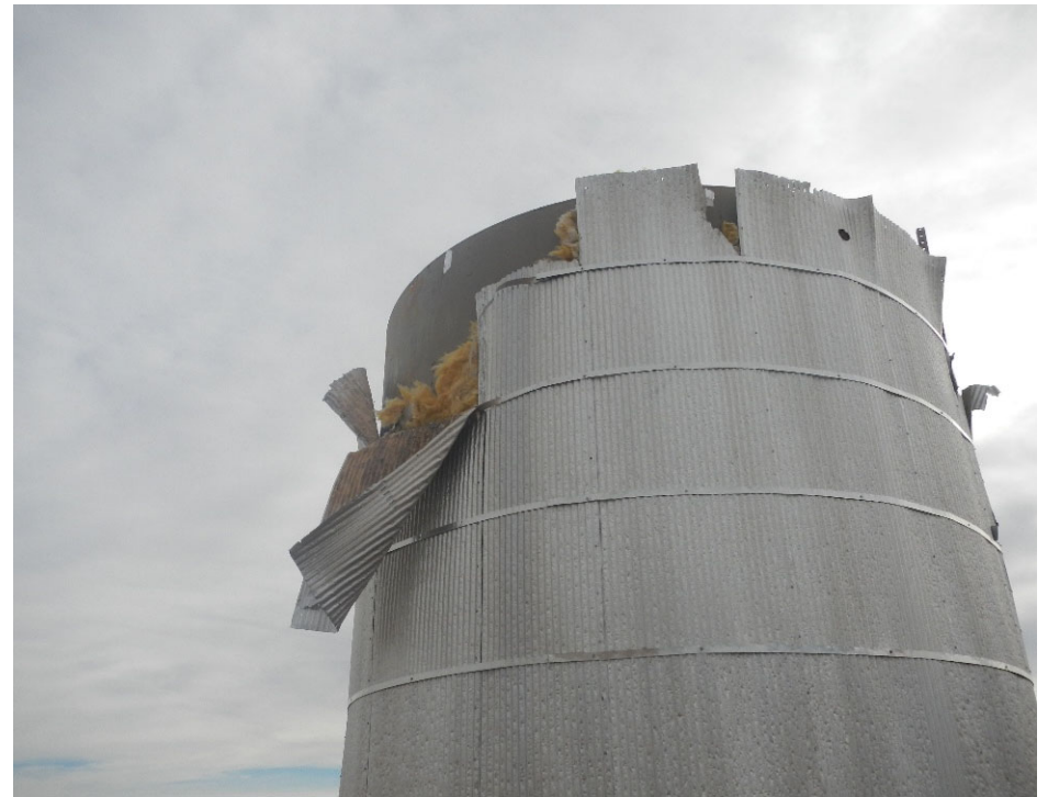
6. View of production tank with insulation visible and metal covering peeling off tank.
