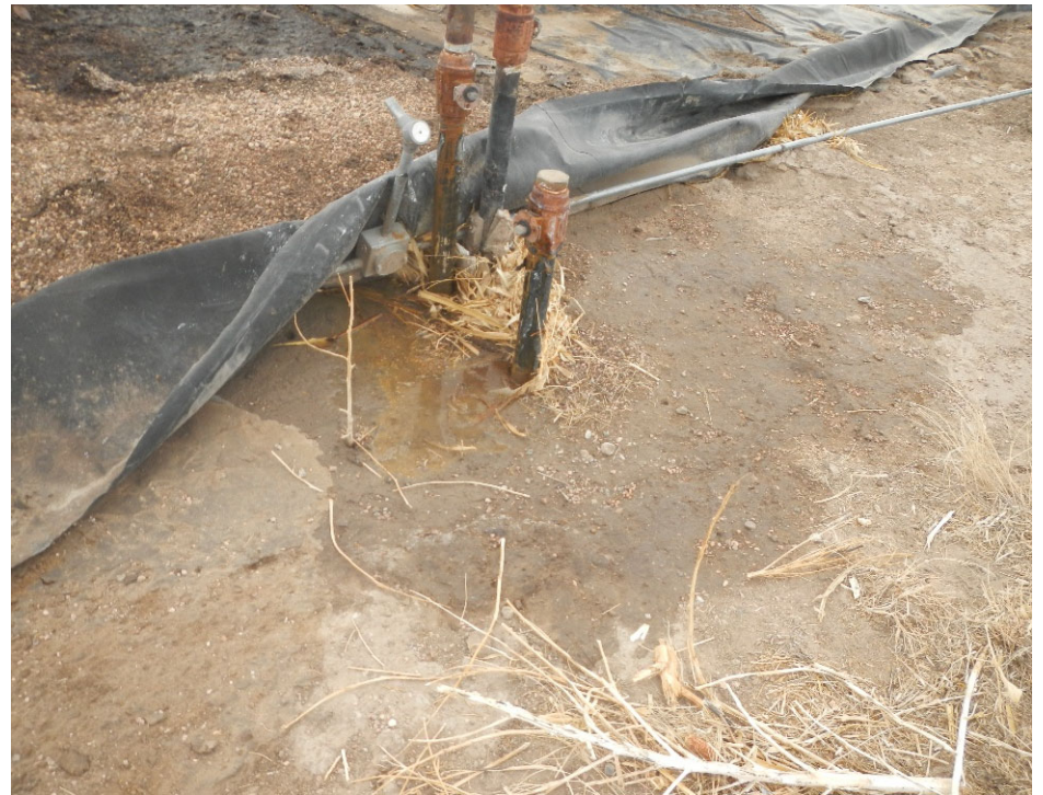
12. Additional view of impacted area with saturated soil under liner.
