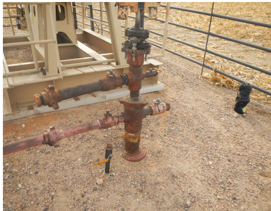
2. View of wellhead. Note one of the three risers at well location right of frame.
