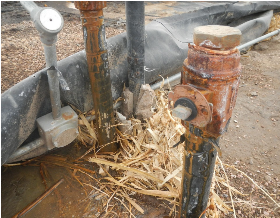
11. Two of two flowline risers leaking from valve body and flowline to valve connection.
