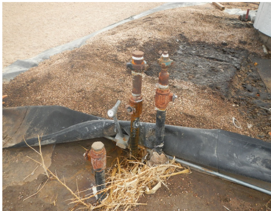
8. View of oily gravel and soil mixture in upper right of frame and flowline risers in center of frame.
