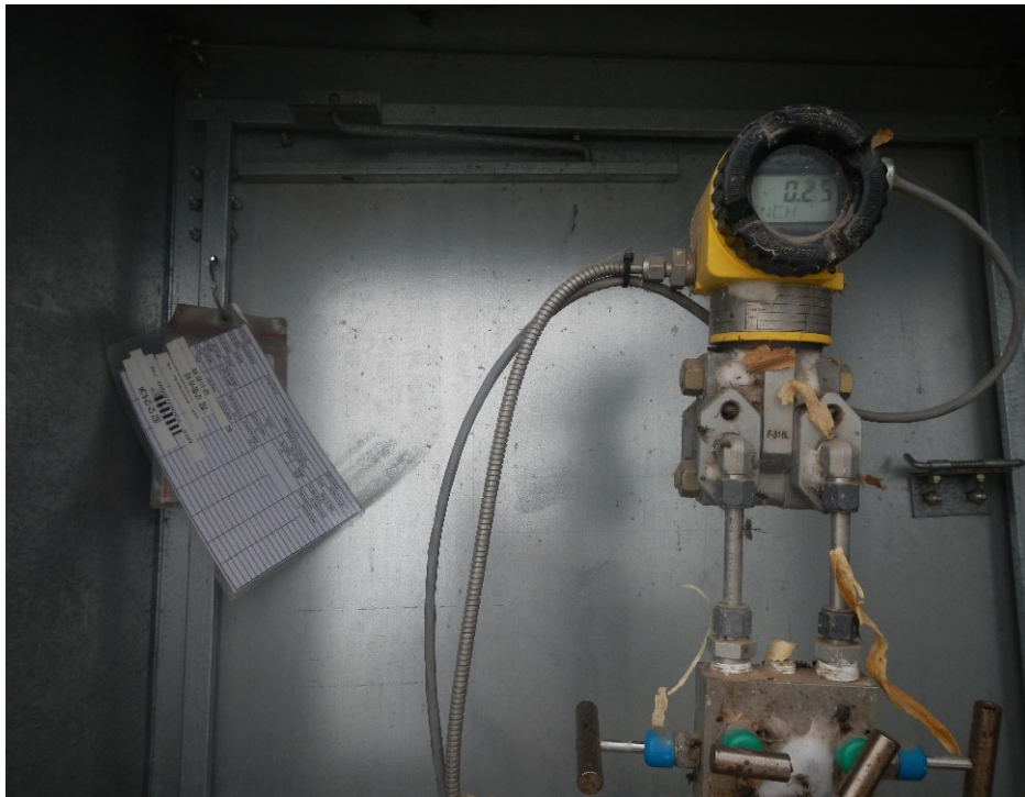
3. Gas Meter inside Flowline mounted Meter Box.
