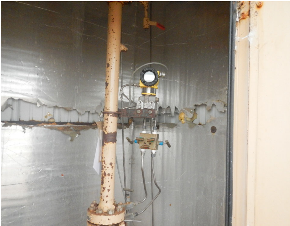
3. Gas Meter inside Meter Shed.
