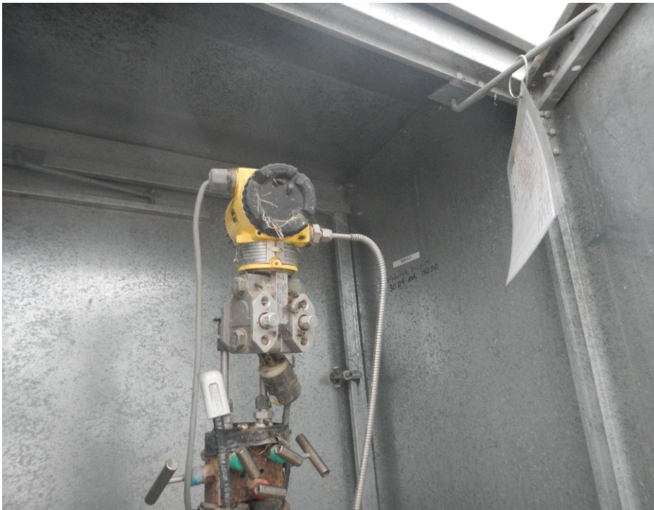
3. Gas Meter inside Flowline mounted Meter Box.
