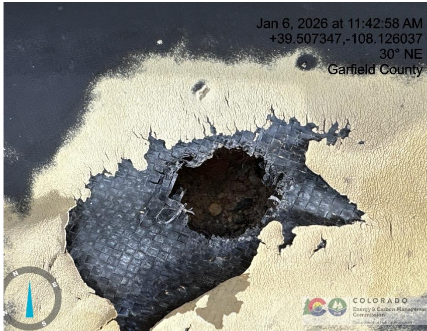
Photo # 8424 Hole in liner/liner needs maintenance
