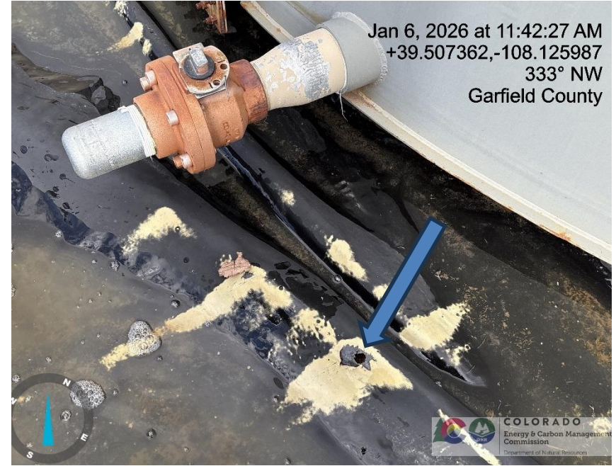
Photo # 8423 Hole in liner/liner needs maintenance
