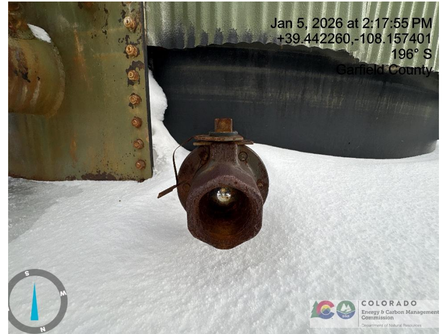
Photo # 8109 Open ended load line
