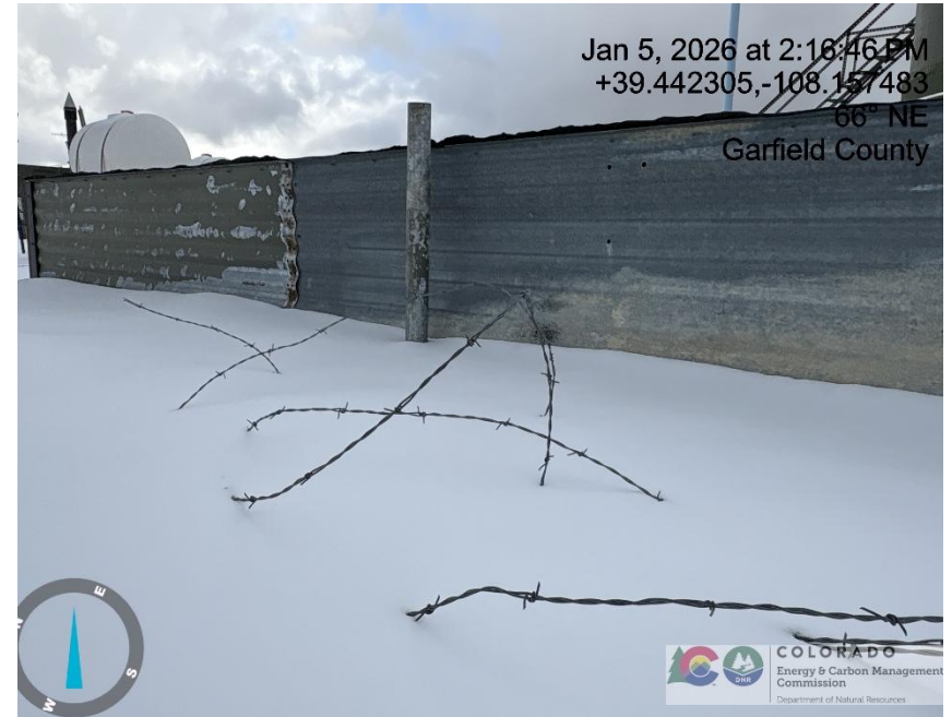
Photo # 8111 Barbed wire fence needs maintenance/wildlife hazard
