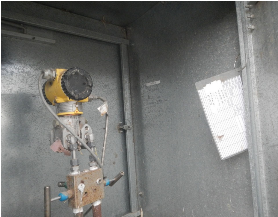
3. Gas Meter inside Flowline mounted Meter Box.
