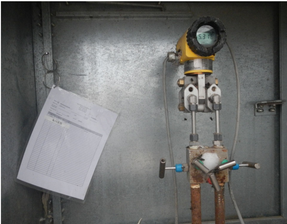
3. Gas Meter inside Flowline mounted Meter Box.
