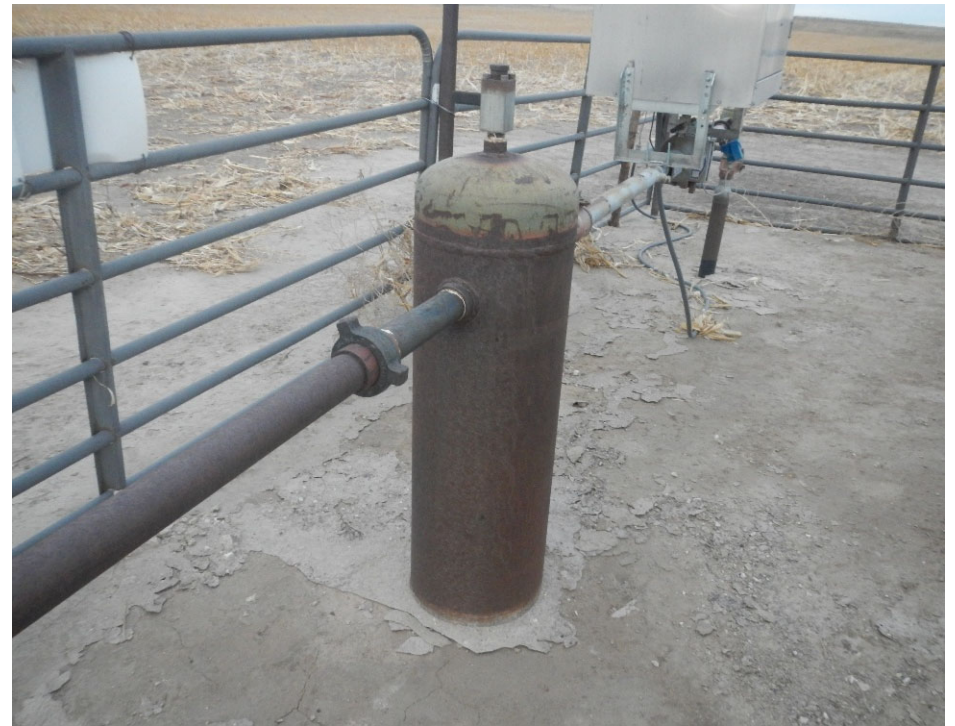
2. View of dehydrator on gas meter inlet.
