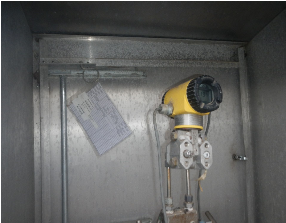
3. Gas Meter inside Flowline mounted Meter Box.
