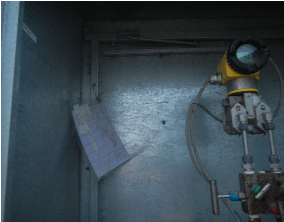
3. Gas Meter inside Flowline mounted Meter Box.
