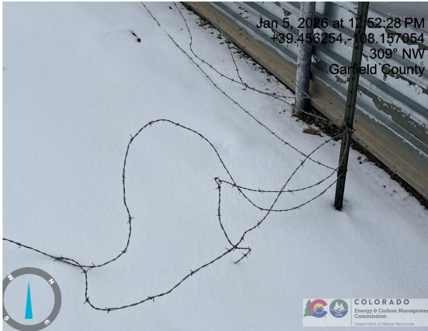
Photo # 7874 Barbed wire fence needs maintenance/wildlife hazard
