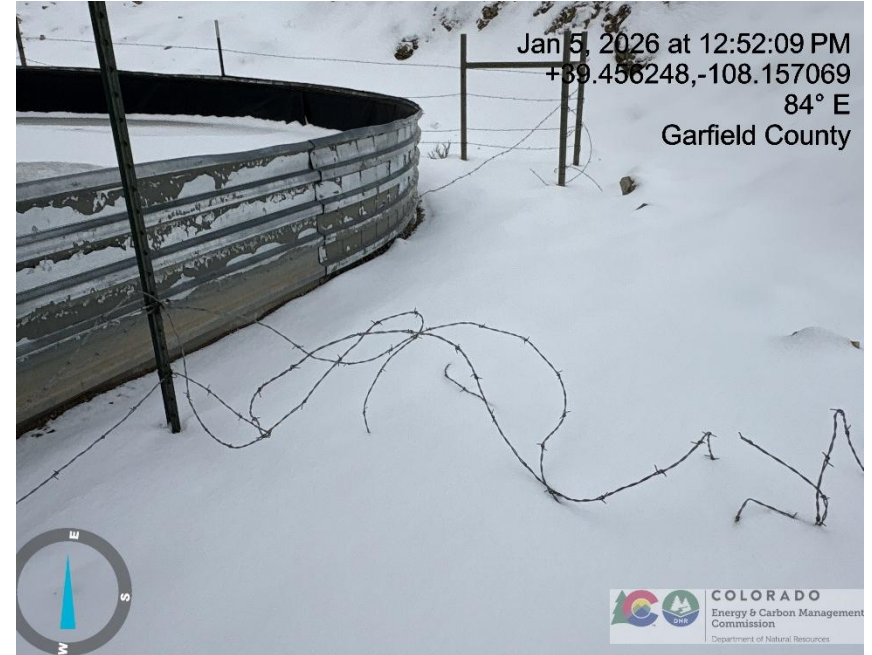
Photo # 7873 Barbed wire fence needs maintenance/wildlife hazard
