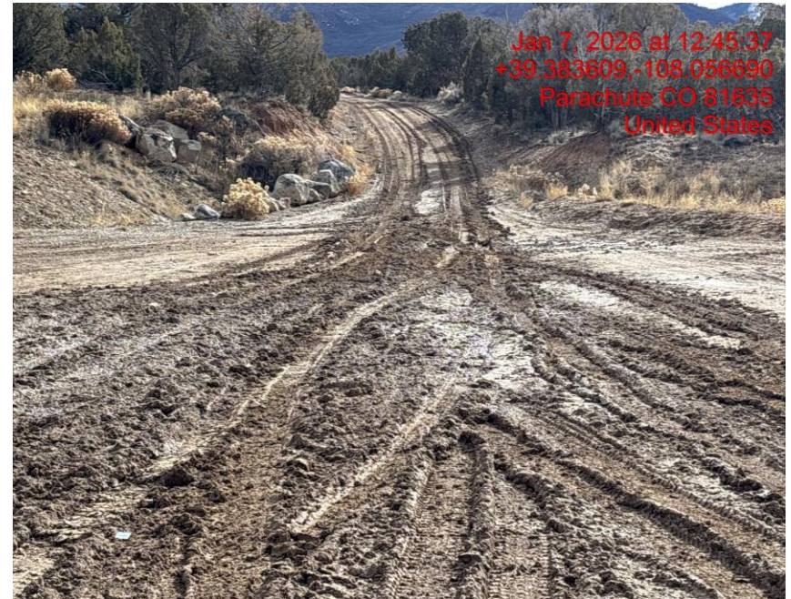
Lack of Stabilization/Insufficient Tracking BMPs – Photo #02239
