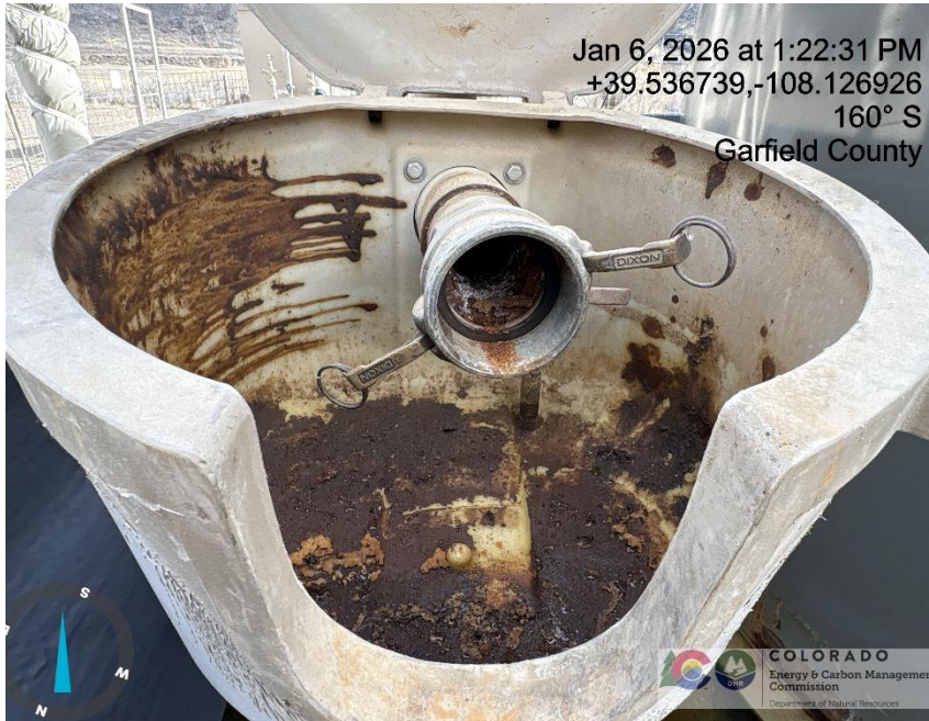
Photo # 8777 Open ended load line
