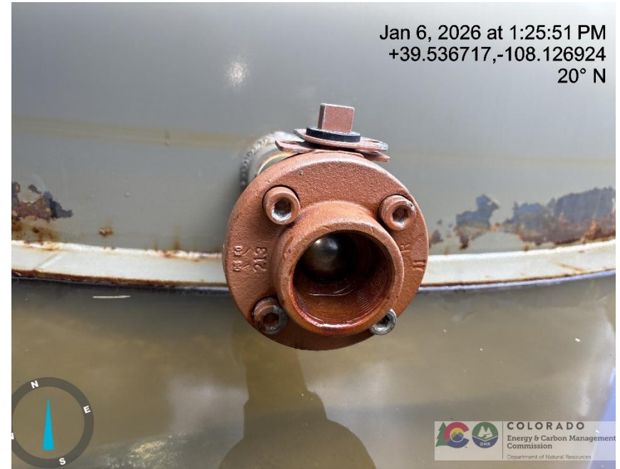
Photo # 8776 Open ended load line
