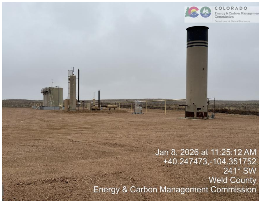
Photo 3 production equipment and tank battery
