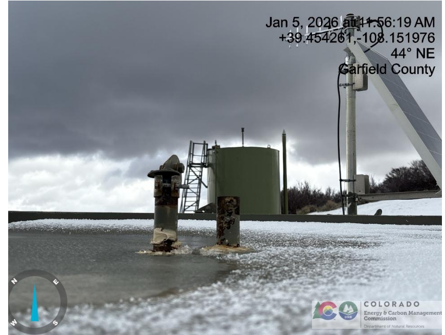
Photo # 7673 Rupture disc vent line does not comply with CECMC pressure safety device rules
