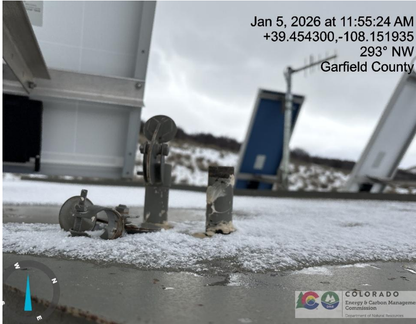
Photo # 7672 PRV vent line does not comply with CECMC pressure safety device rules
