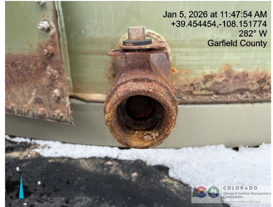
Photo # 7671 Open ended load line
