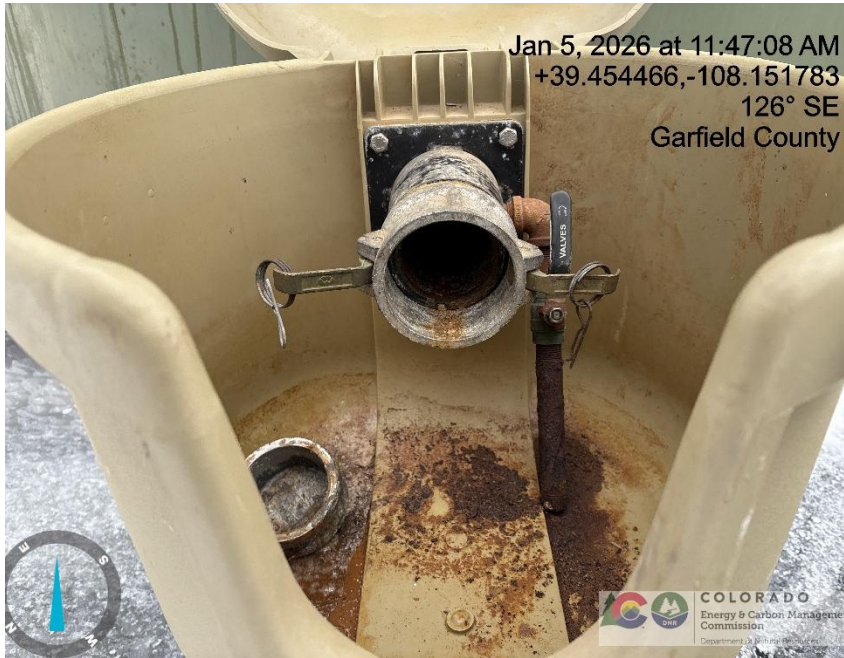
Photo # 7670 Open ended load line
