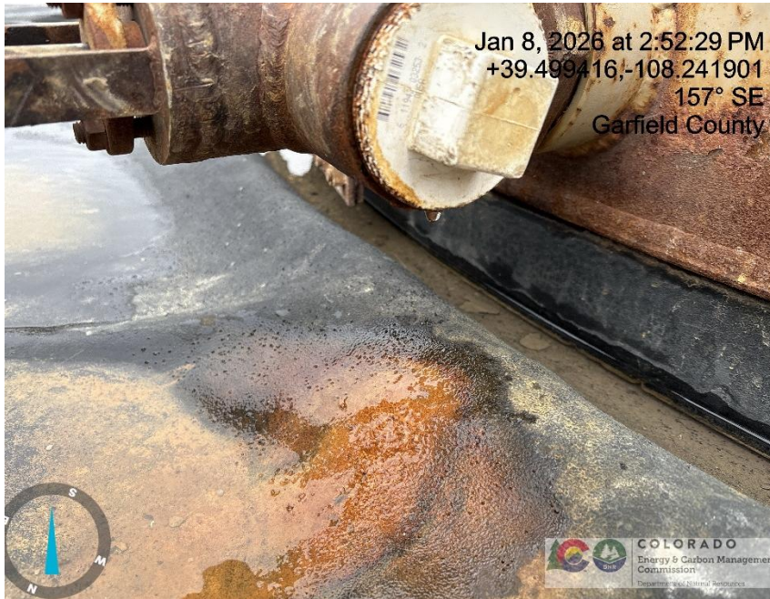
Photo # 9659 Mechanical Condition - Possible leak on tank valve
