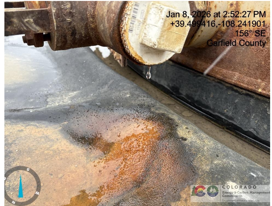
Photo # 9660 Mechanical Condition - Possible leak on tank valve
