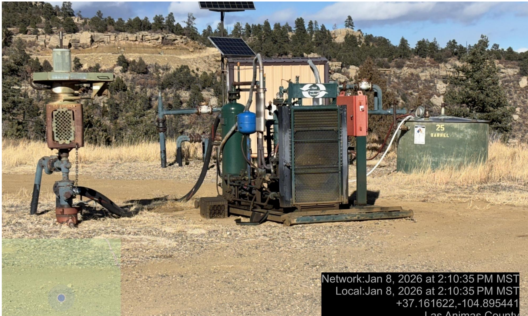
PHOTO 5: CH WELLHEAD AND EQUIPMENT./ Vacuum pump observed on CH well without ECMC approval. Provide ECMC with documentation showing approval of use of vacuum pump. CA DATE 1/26/2026.
