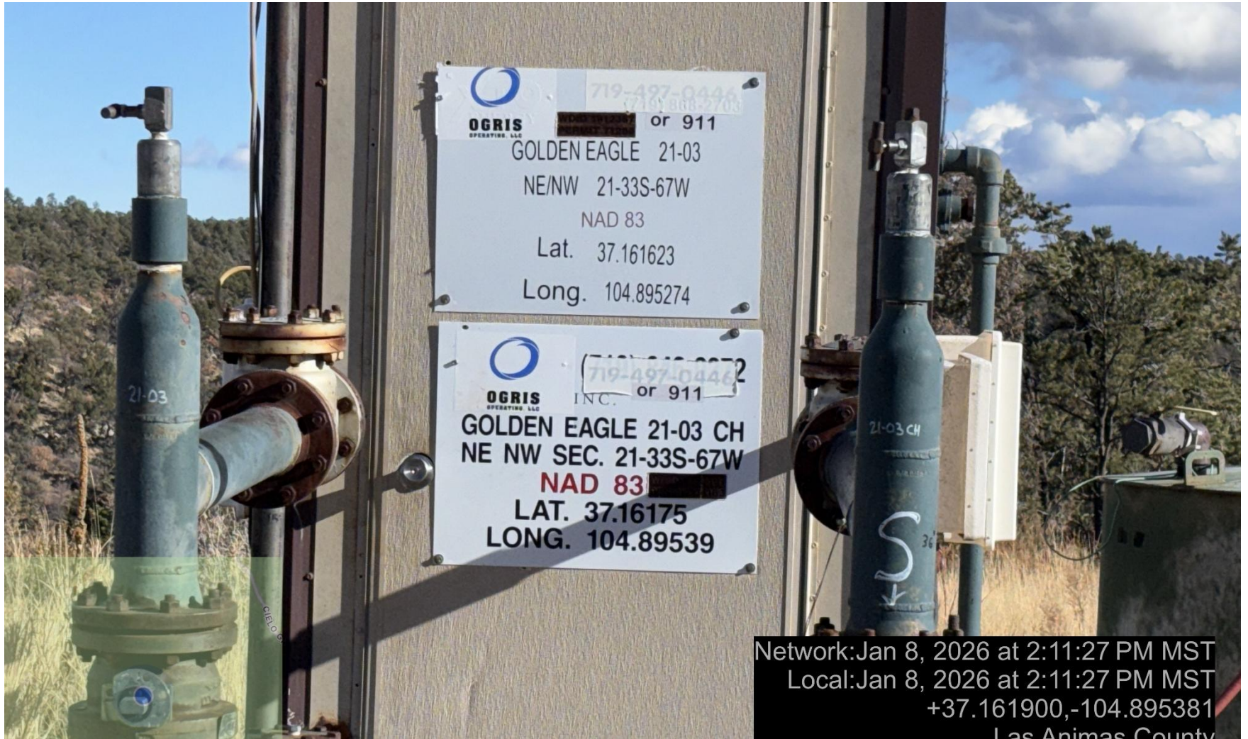
PHOTO 2: API # IS NOT POSTED ON EITHER WELL SIGNS.
