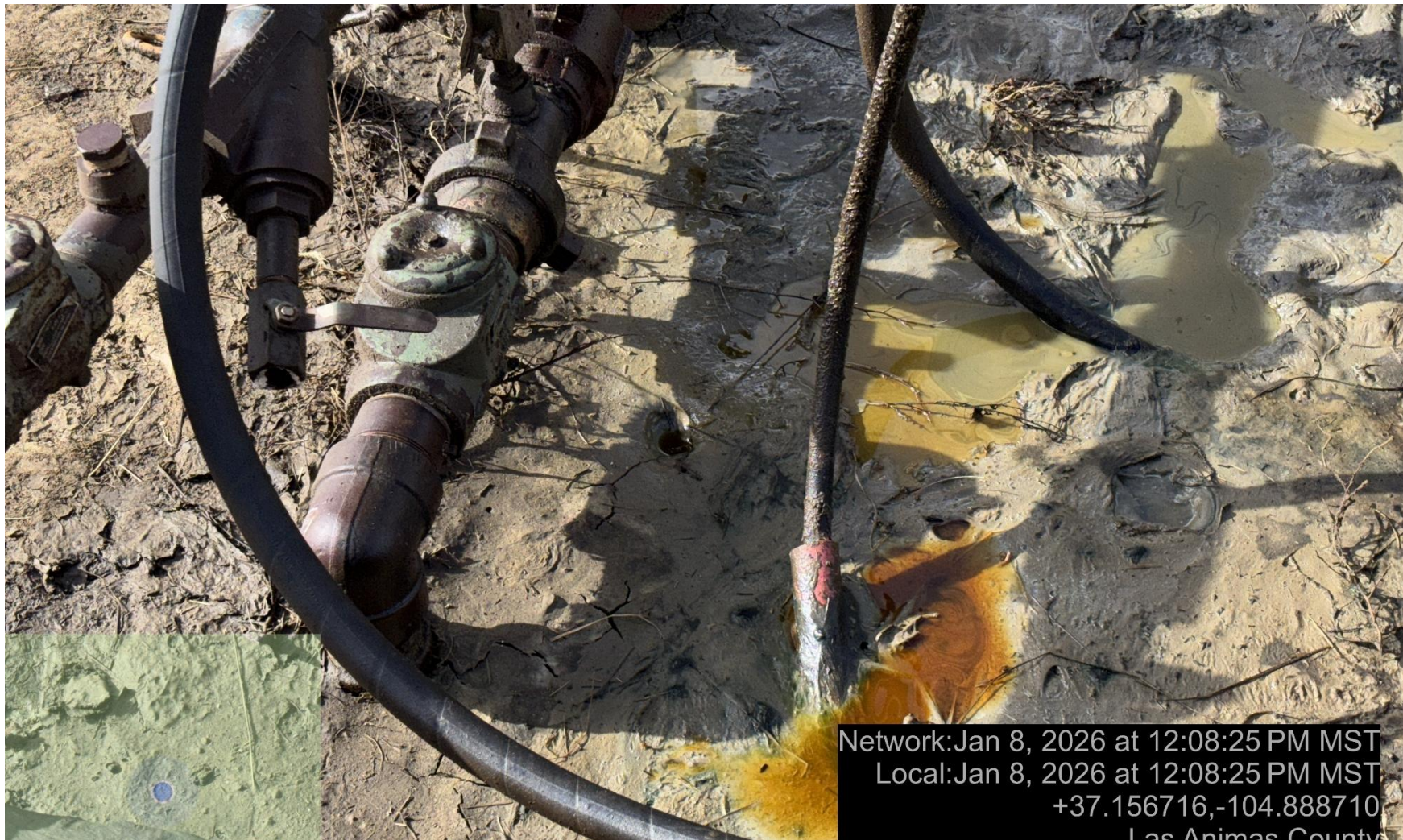
PHOTO 5: There is a dripping leak at the wellhead and a pool of water at wellhead with an oily sheen. Control and contain spills/releases and clean up per Rule 912.a. THIS IS THE SECOND NOTICE FOR THIS CA IMMEDIATE ACTION IS REQUIRED.
