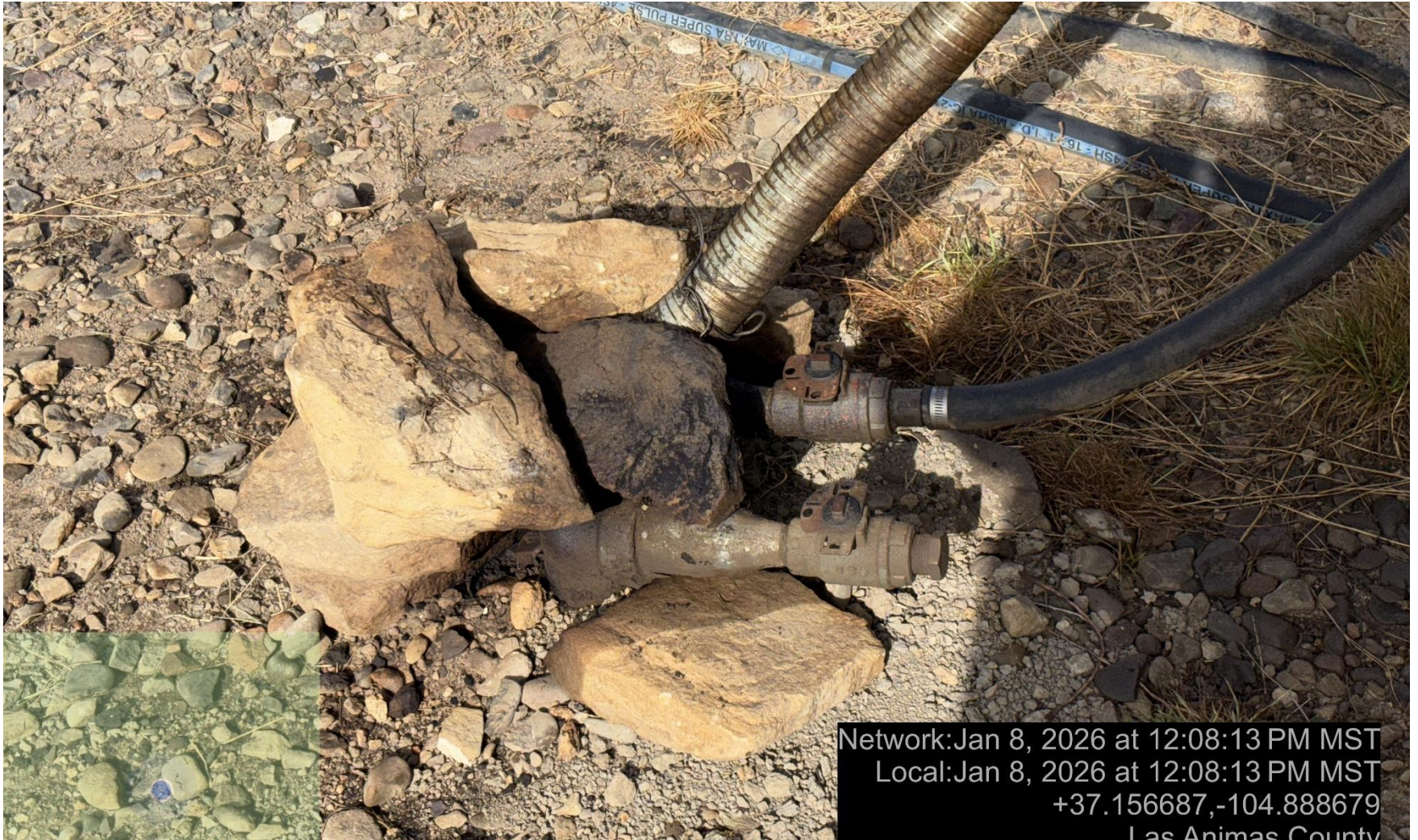
PHOTO 6: There is oily fluids in the engine skid and stained material at the engine exhaust pipe. Conduct maintenance on equipment, cleanup stained material and review self inspection processes. THIS IS THE SECOND NOTICE FOR THIS CA IMMEDIATE ACTION IS REQUIRED.
