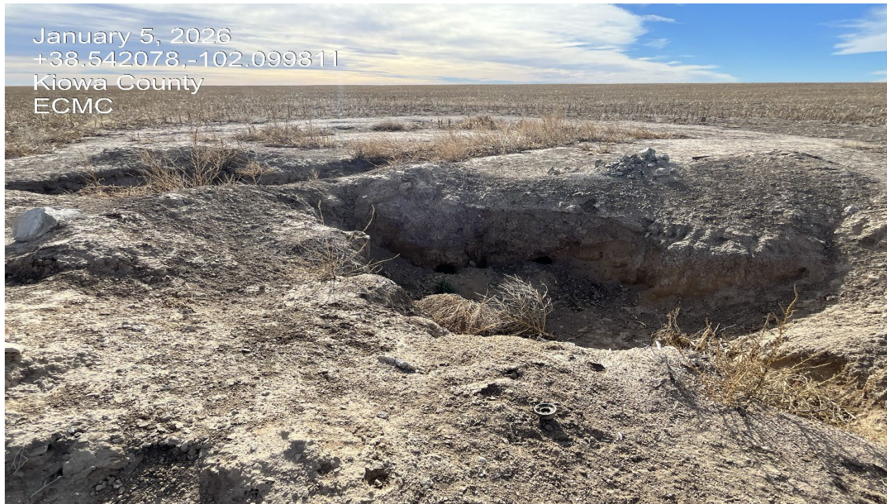
Photo 2. Facing south toward the abandoned wellsite. An open excavation remains at the location.
