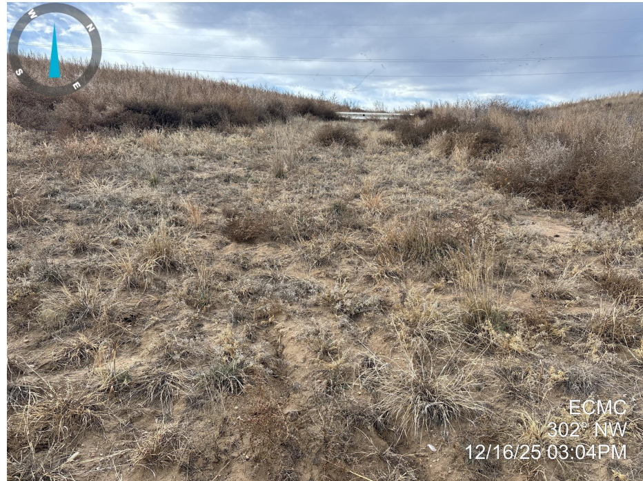
Photo 6. Photo taken of the access road to the location, facing northwest, towards the location. Stormwater erosion was observed along the southeastern portion of the road.
