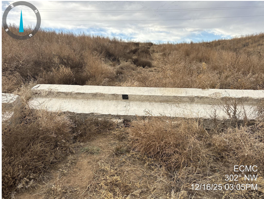
Photo 5. Photo taken of the access road to the location, facing northwest, towards the location. Photo illustrates that final reclamation activities have taken place, but vegetation has not established to Rule 1004 standards. A concrete barrier has been implemented along the access road.
