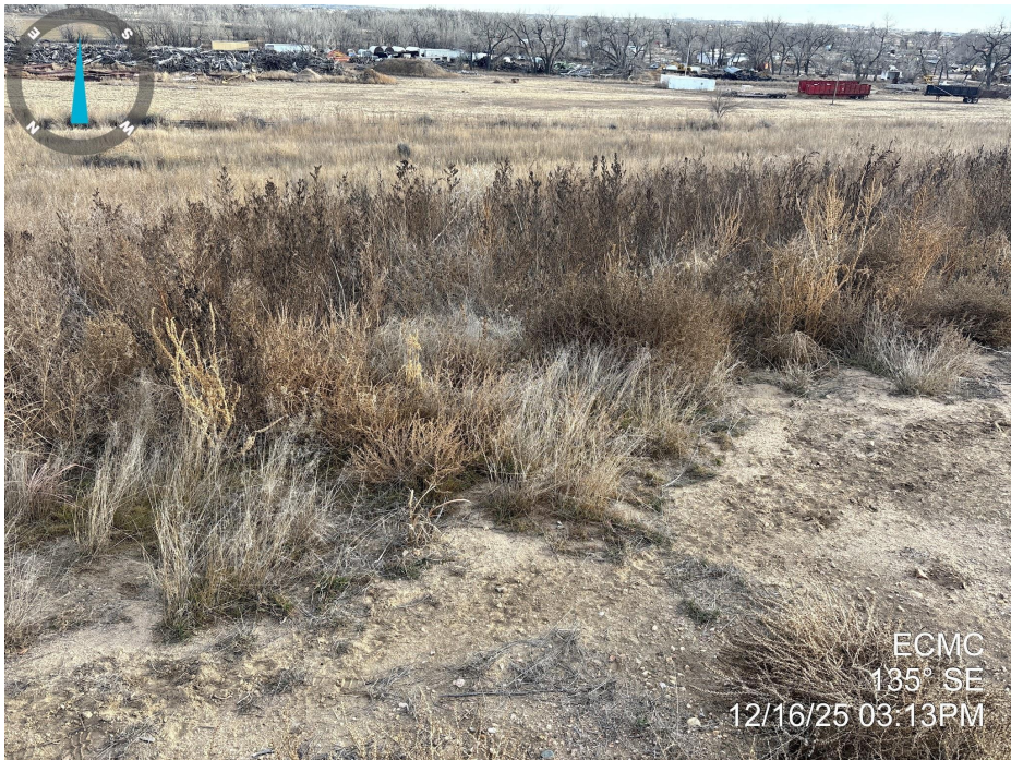
Photo 7. Photo taken of the tank battery location, facing southeast. Photo illustrates that final reclamation activities appear to have taken place, but the location does not meet Rule 1004 standards as weedy annual vegetation was observed across the location.
