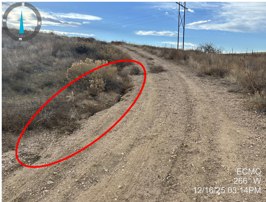
Photo 6. Photo taken of the access road to the location, facing west, towards the location. Stormwater erosion was observed along the edge of the road (highlighted in red).
