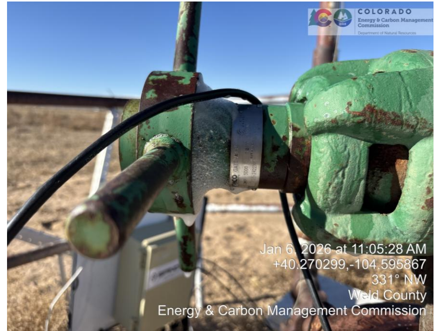
Photo 2 well head master valve leaking
