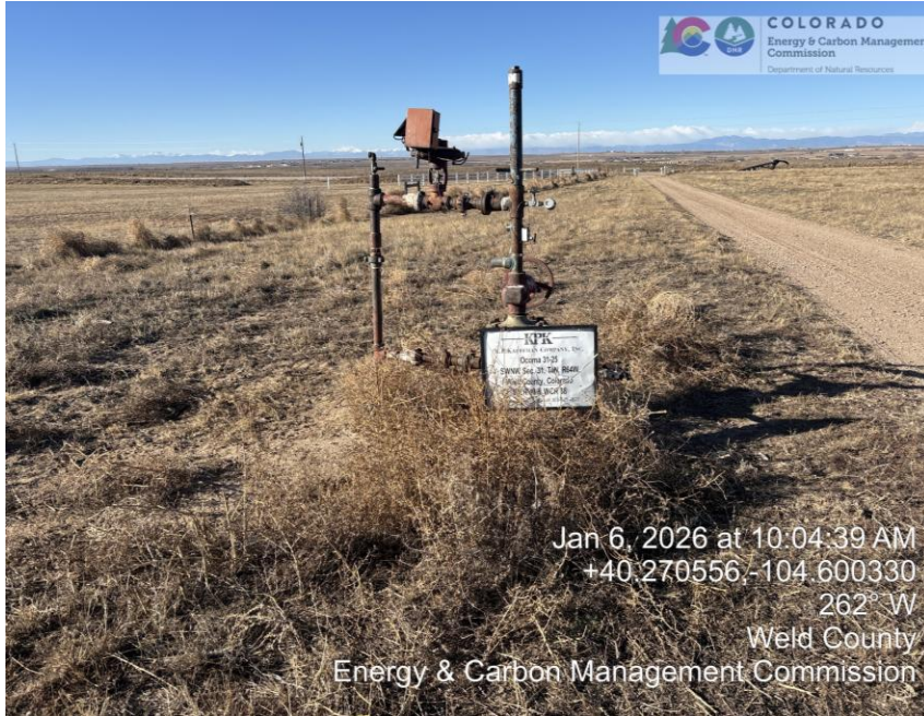
Photo 1 well head and equipment
