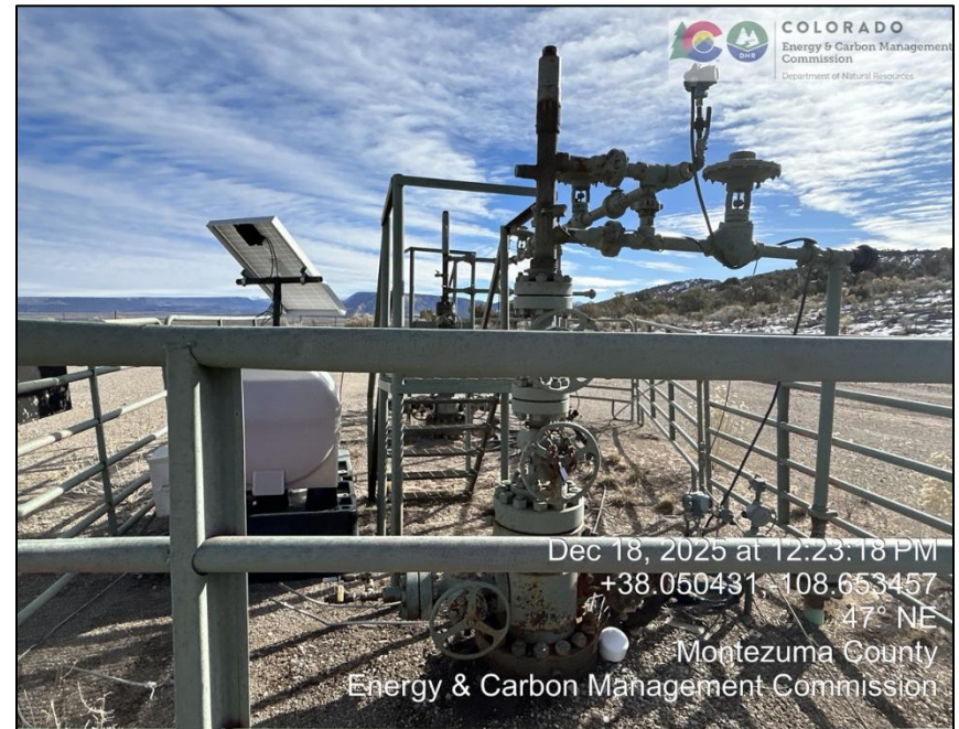
06.) Andy's Mesa Federal 67 (foreground) and 66 (background). Note that injection (methanol?) system is hooked up to non-functioning equipment and is non-functional itself. Secondary containment appears to be about half full of water.
