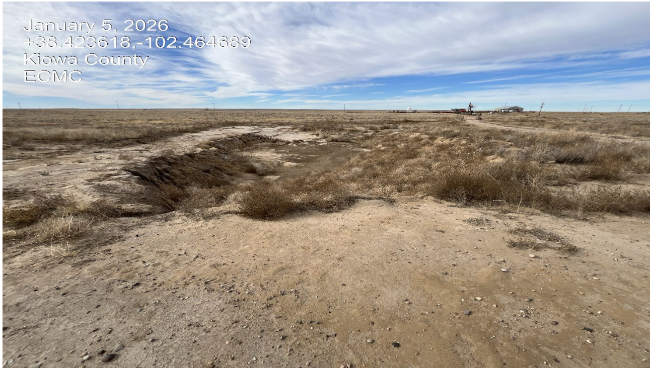
Photo 3. Facing east toward the remediation excavation area. Remediation remains in process and has been ongoing since 2022. There is undesirable weed debris accumulated inside the excavation.
