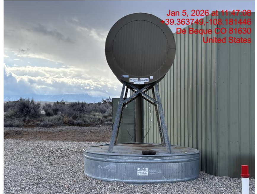
Location/Unsecured Secondary Containment – Photo #02203
