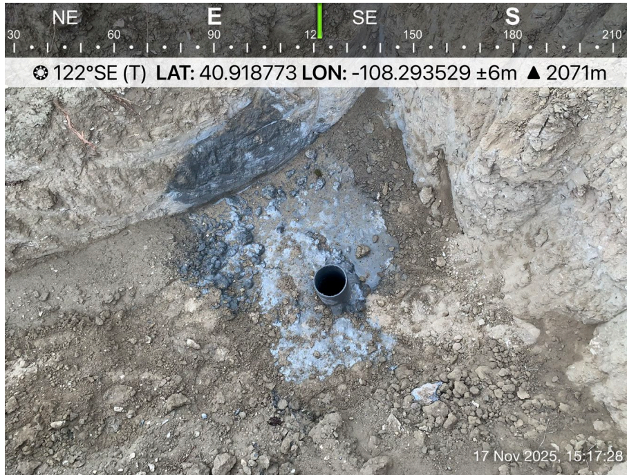
Photo 1: State #31-16 (OWP) P&A well, view from above, no methane detected.
