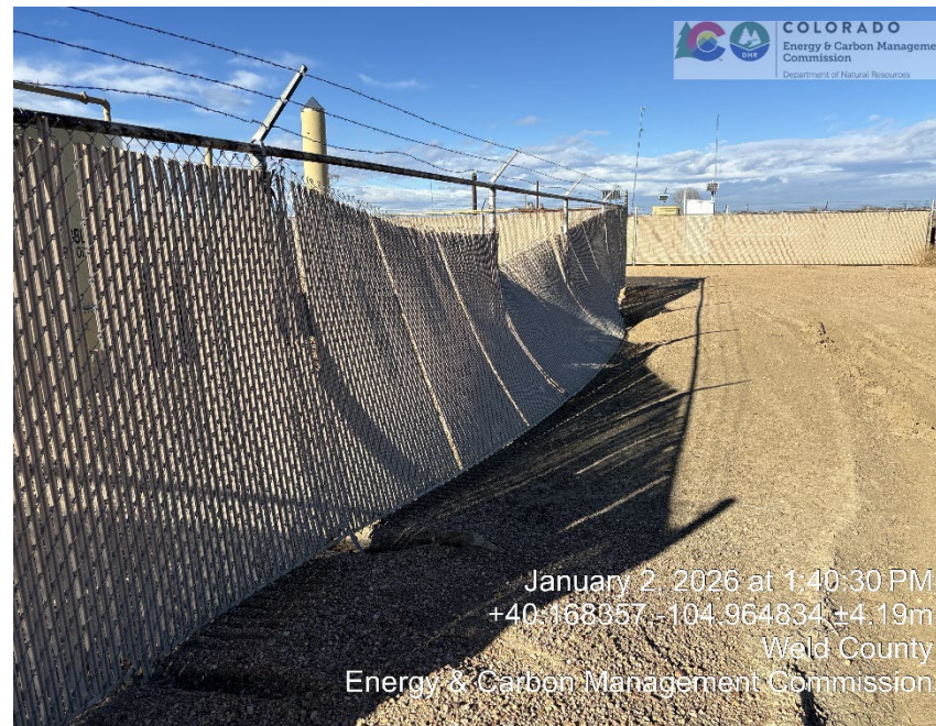
East crude oil tank fencing
