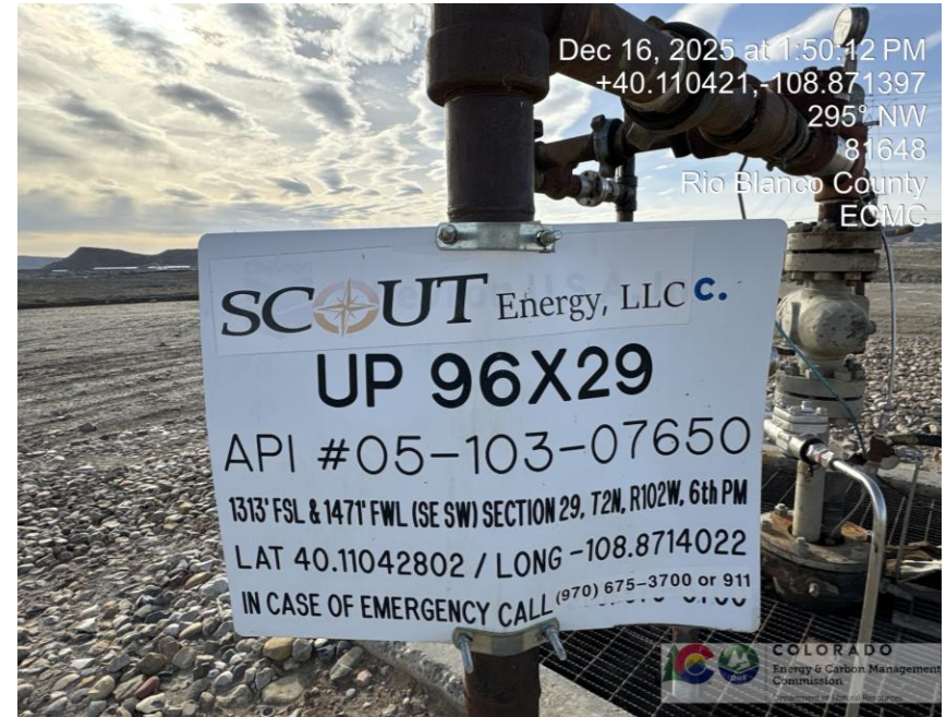
Photo # 0323 Wellhead sign lacks public road used to access the well
