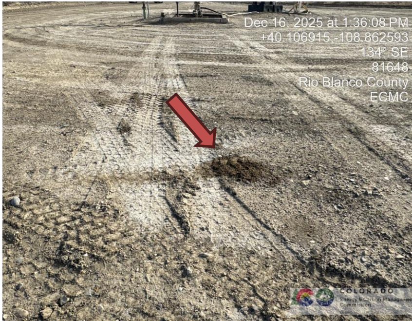
Photo # 0303 Staining on location
