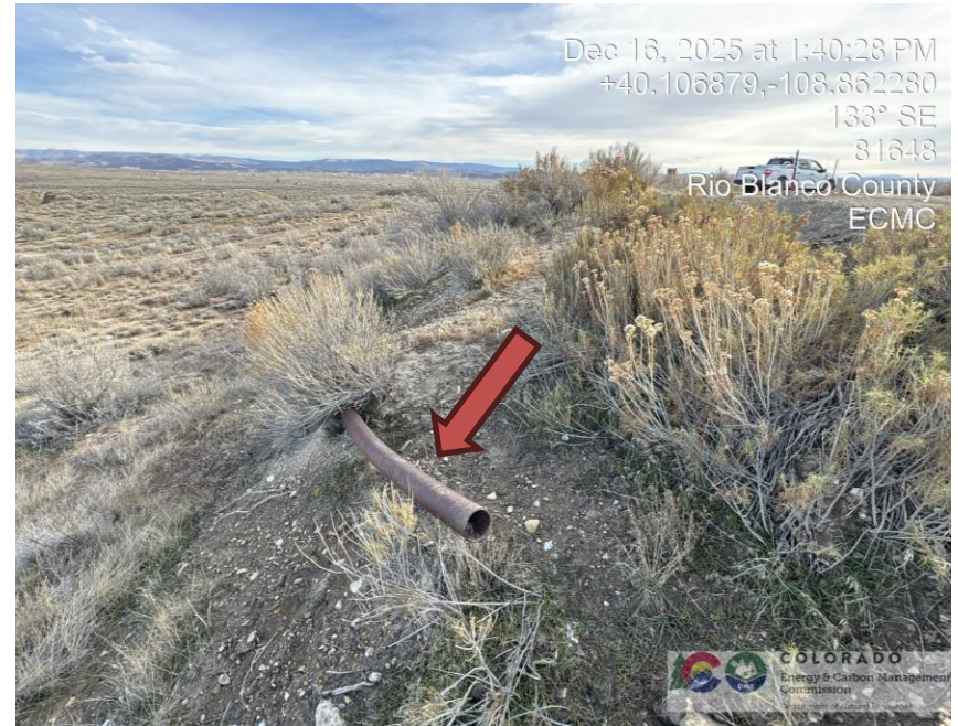
Photo # 0308 Debris on NE side of location
