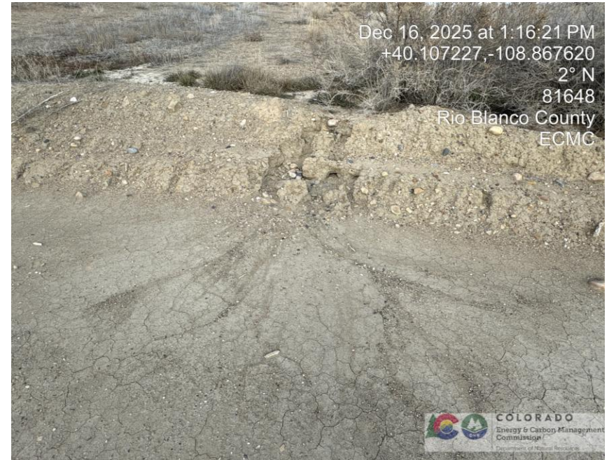
Photo # 0280 Loss of berm integrity due to erosion on north side of location/insufficient BMP's
