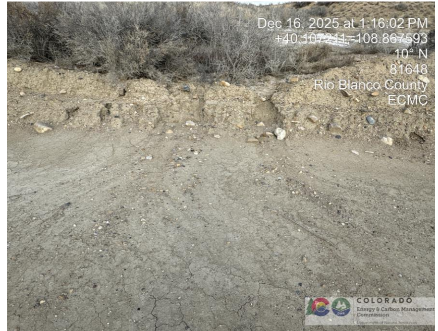
Photo # 0277 Loss of berm integrity due to erosion on north side of location/insufficient BMP's
