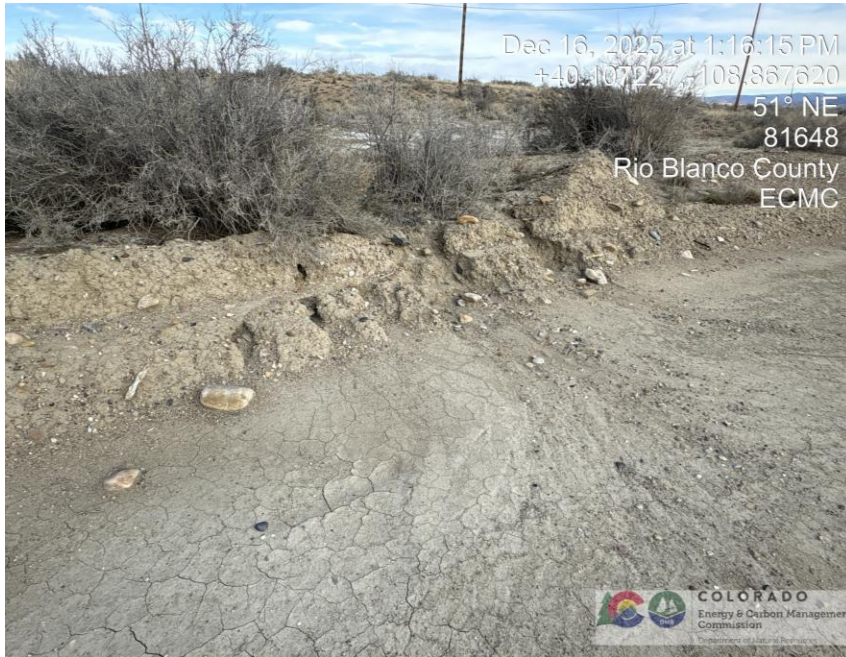
Photo # 0279 Loss of berm integrity due to erosion on north side of location/insufficient BMP's
