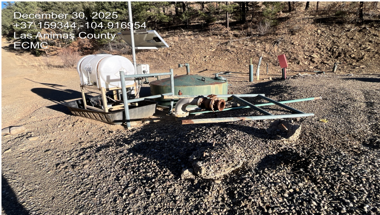
Photo 3. There are tanks and risers that don't appear to be needed or in use and must be removed.
