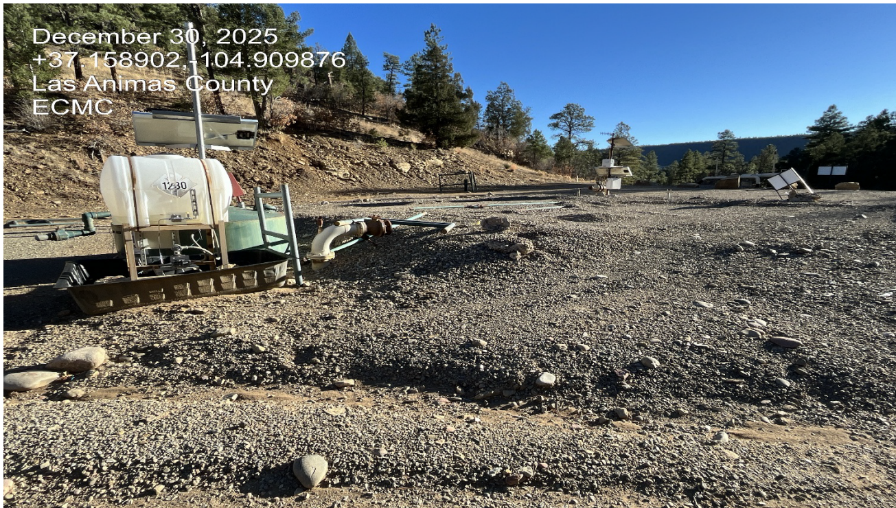
Photo 1. Facing southwest toward the GE 9 compressor station. The compressor has been removed.
