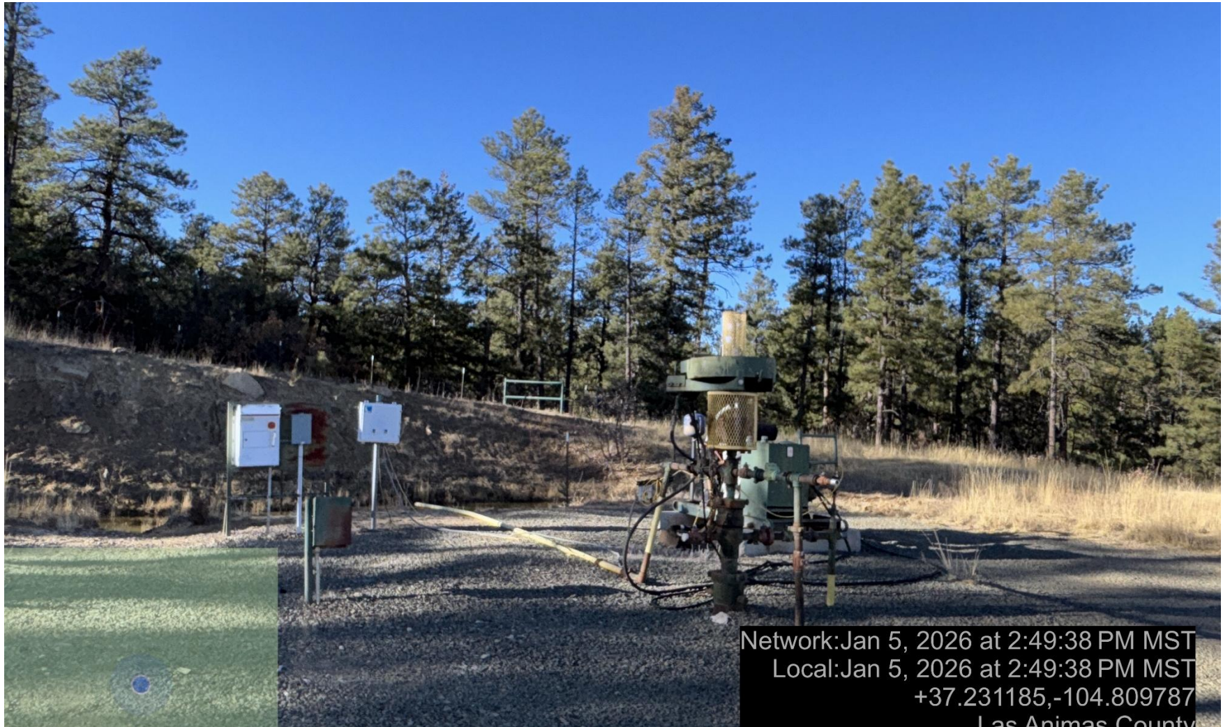
PHOTO 4: WELLHEAD AND EQUIPMENT.
