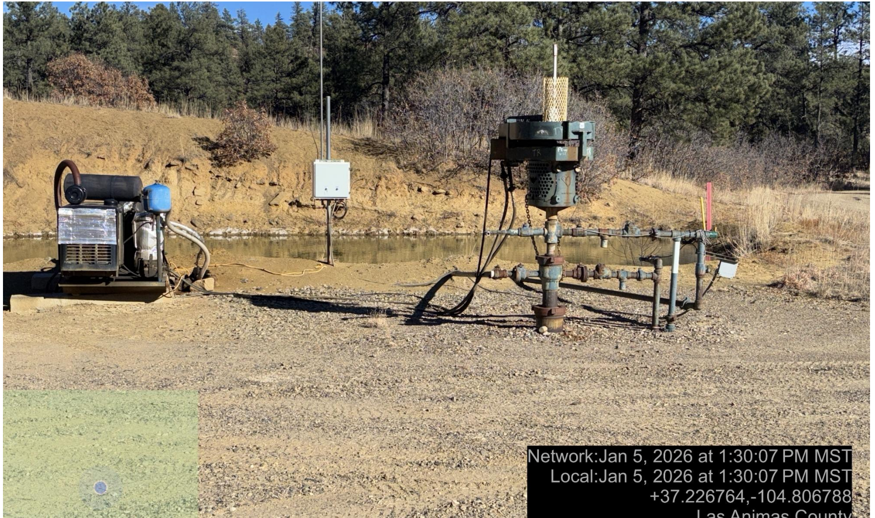
PHOTO 5: TR WELLHEAD AND EQUIPMENT.
