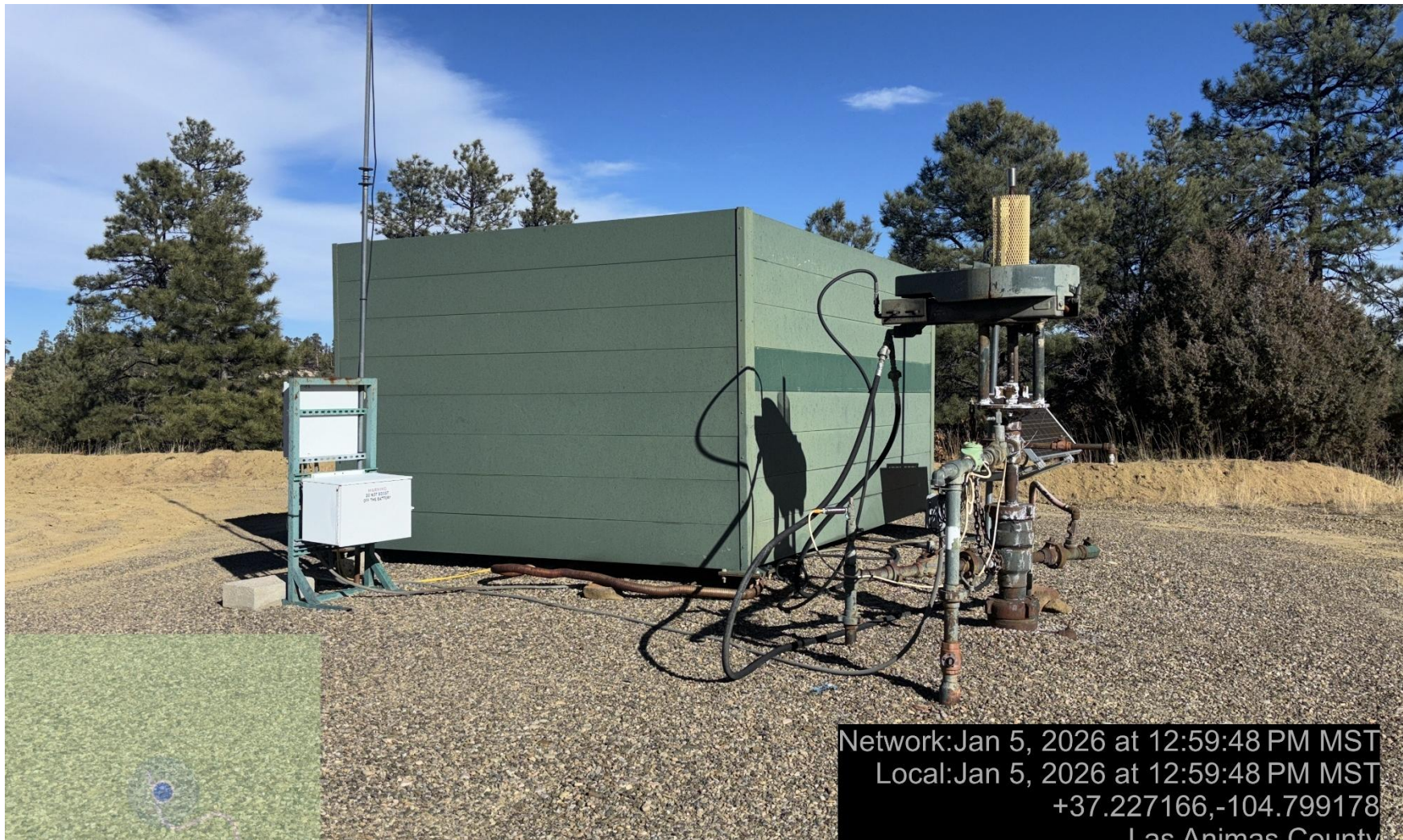
PHOTO 4: KVWELLHEAD AND EQUIPMENT.
