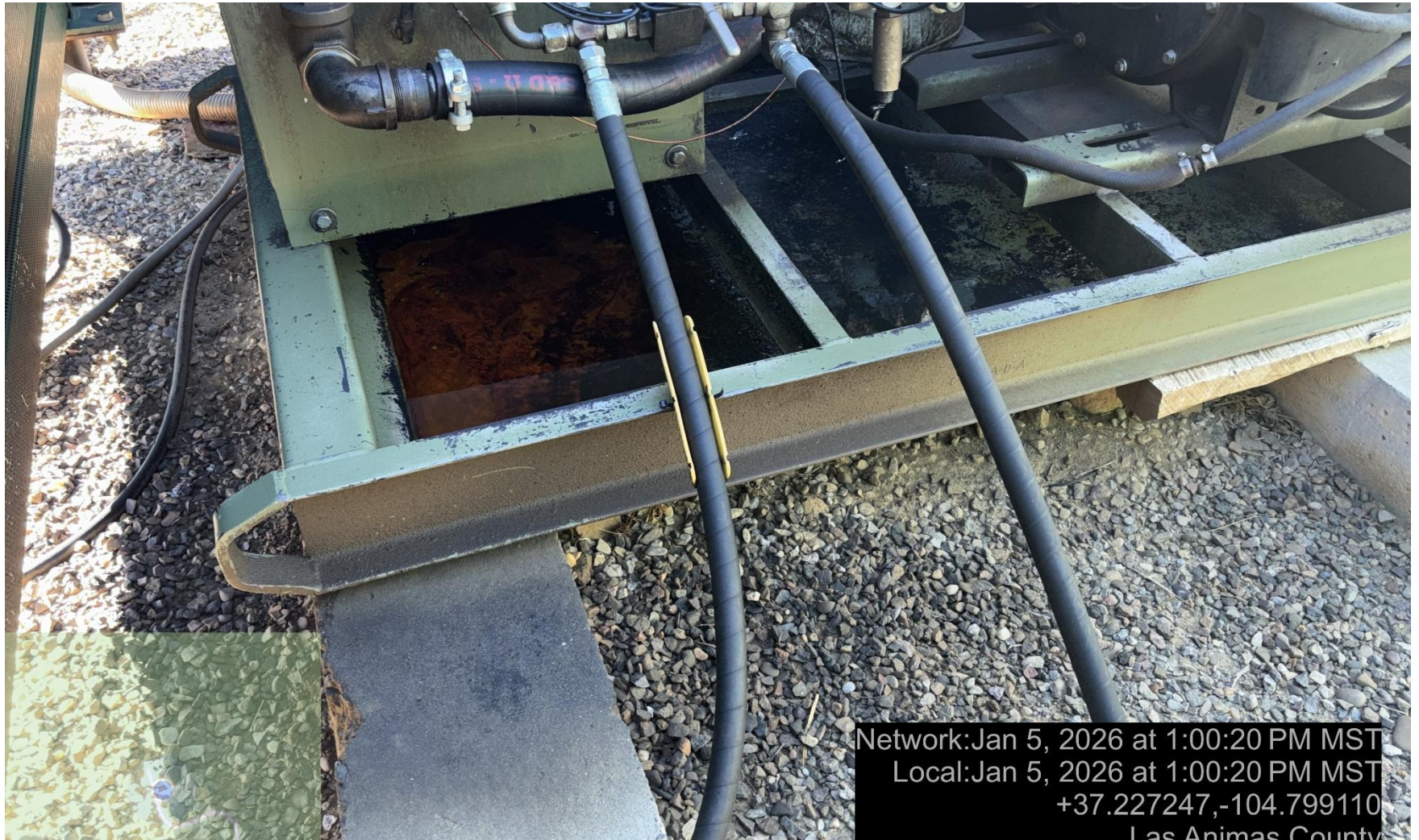
PHOTO 5: OILY WASTE IN PRIME MOVER ENGINE SKID. DRAIN OILY WASTE REPAIR ALL LEAKS AND REMOVE IMPACTED SOIL PER RULE 1002..(2).D & 1002.f.(2)B, Comply with general provisions of the oil and gas act for wildlife protection AND SB-181. 24 HOURS TO DRAIN OILY WASTE 1/6/2026, 10 DAYS TO REMOVE IMPACTED SOILS. 1/16/2026.
