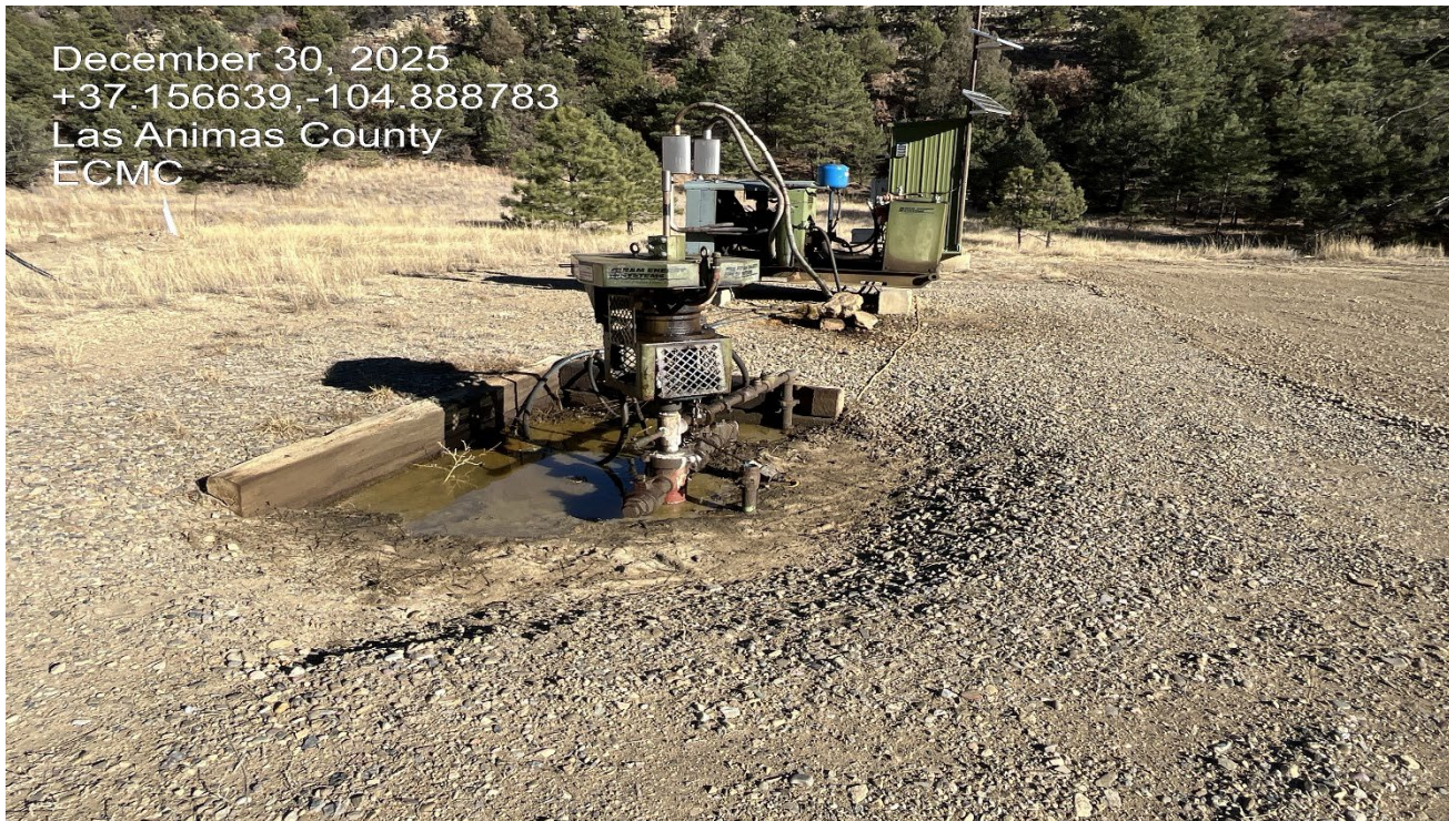
Photo 2. Facing toward the wellhead. There is a dripping leak at the well and standing water appears to have oily fluids comingled.
