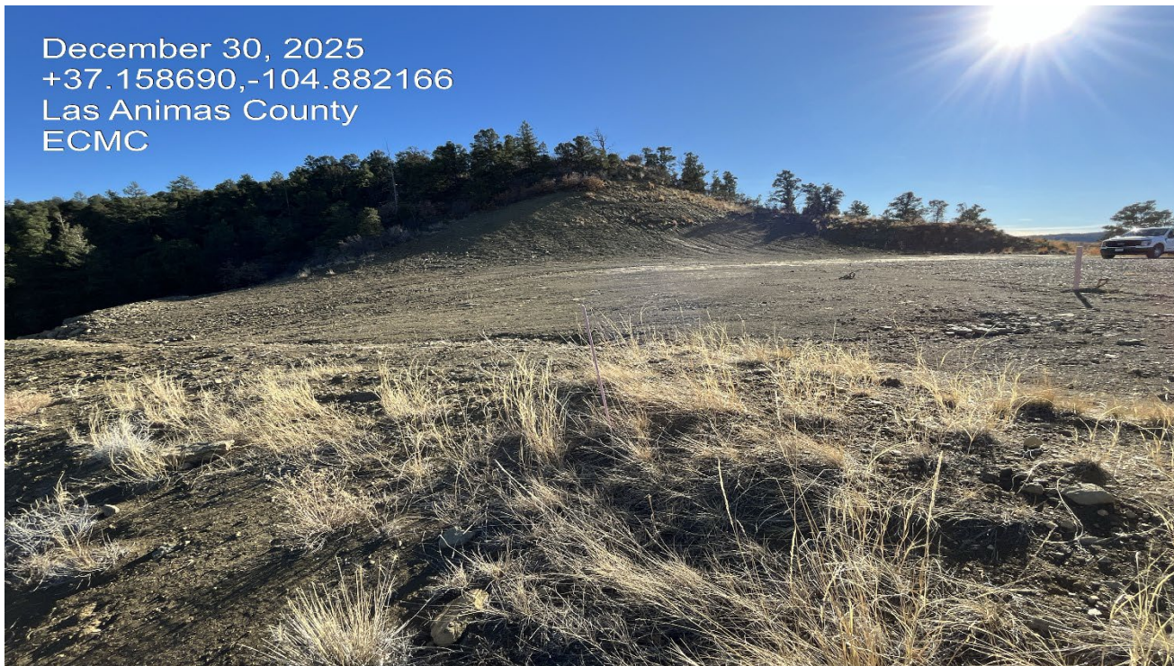
Photo 3. Facing southwest at the location. The fill slope will need to be recontoured back into the original contours to comply with 1004 Rules.
