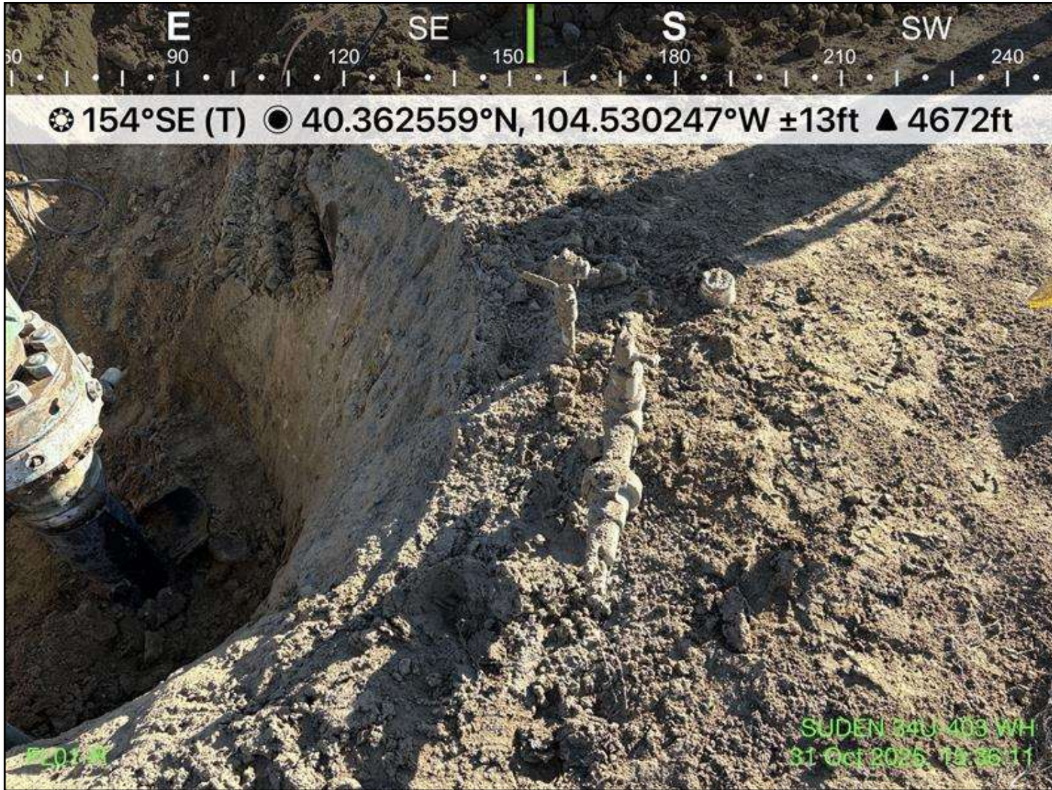
Photo 3: View of flowline riser, facing southeast
