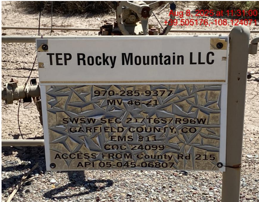
Illegible Wellhead Sign – Photo #00075 From inspection/audit 719500308 conducted on 08/08/2025
