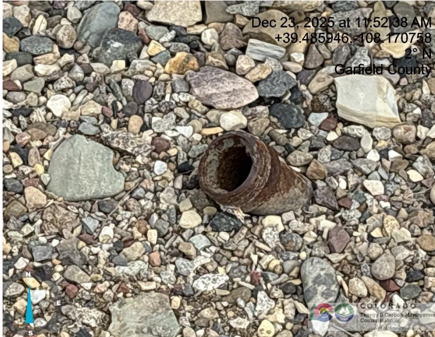
Photo # 5472 Open ended piping near wellhead/wildlife hazard/available for entry by wildlife
