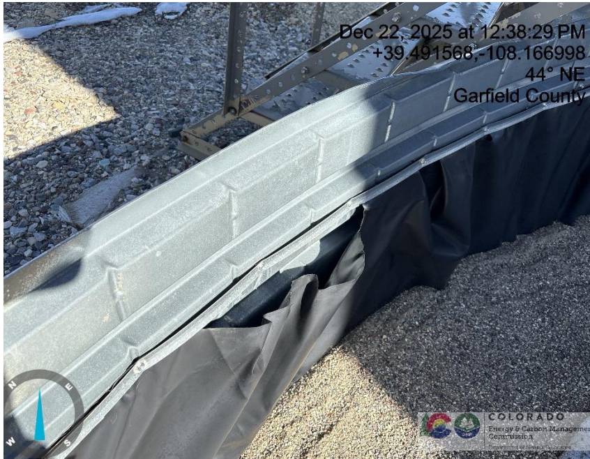
Photo # 4971 Secondary containment liner damaged/liner needs maintenance
