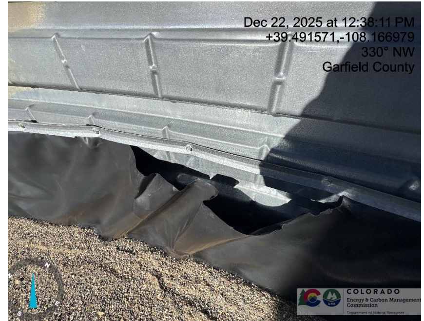
Photo # 4972 Secondary containment liner damaged/liner needs maintenance
