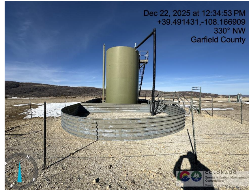
Photo # 4970 Battery lacks required signage
